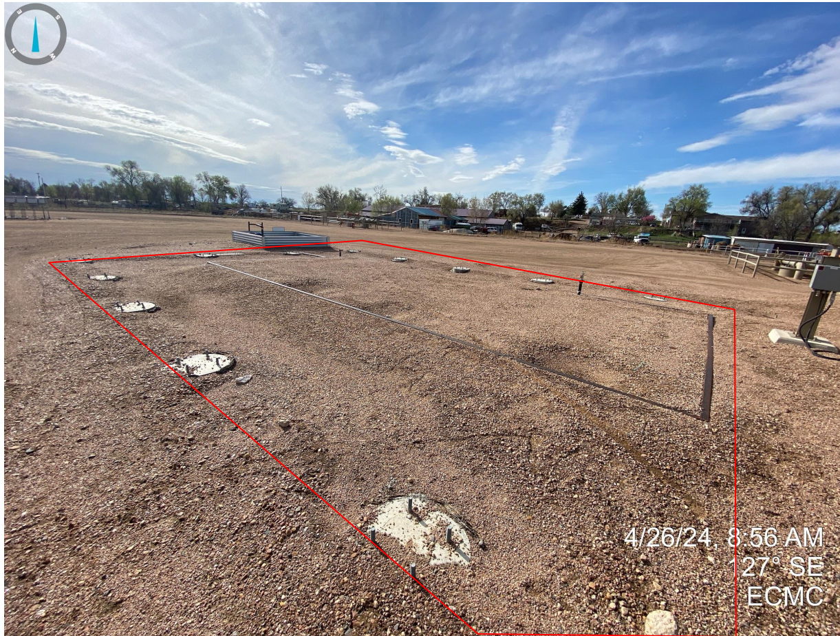
Photo 2. Former compressor location; unused equipment identified in the red polygon must be returned to service or removed from the location.
