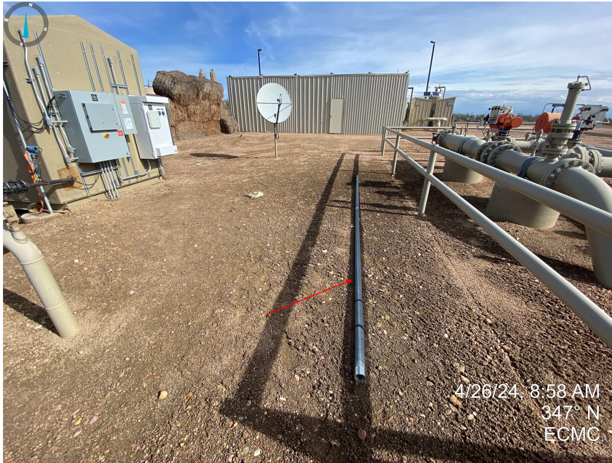
Photo 6. Unused equipment south of compressor station must be returned to service or removed from the location.
