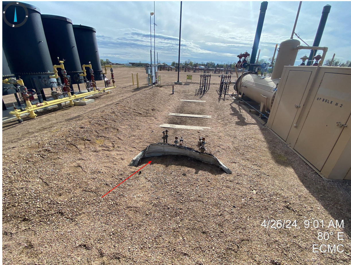
Photo 12. Debris/trash observed within equipment.
