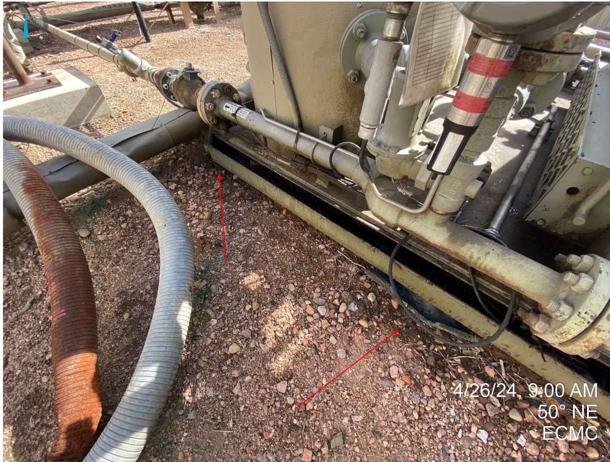
Photo 10. Stained soil at compressor station.
