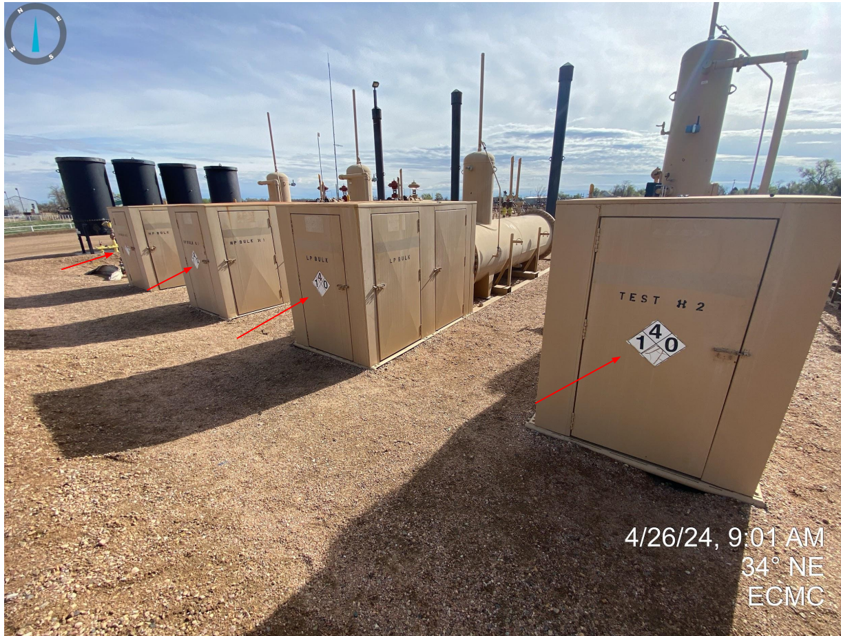
Photo 11. Equipment labels are faded, peeling, cracked.
