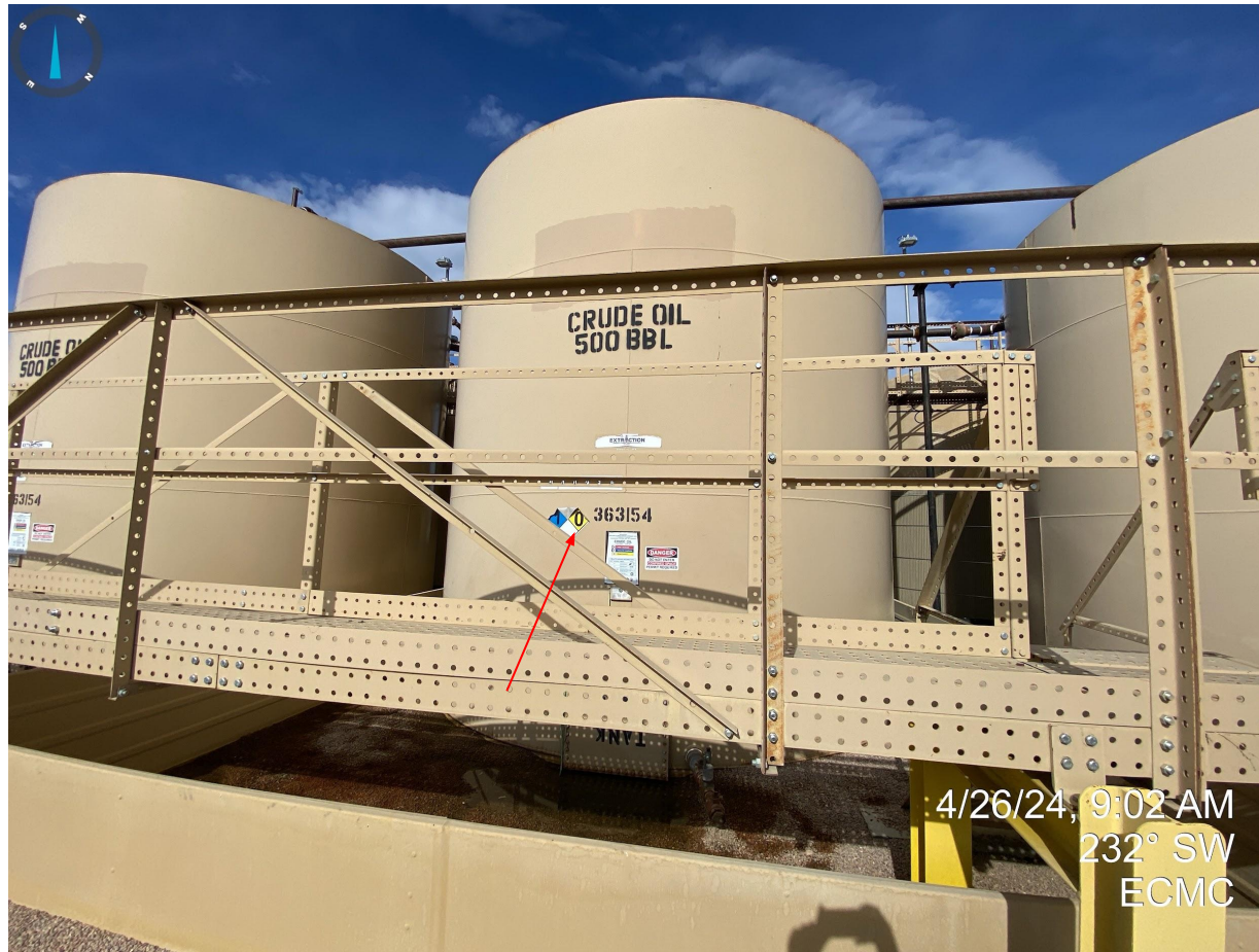
Photo 13. Tank labels/NFPA placards are faded, peeling, cracked.
