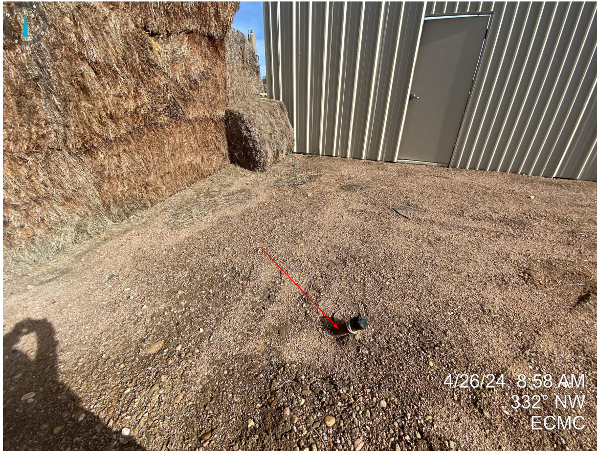
Photo 5. Unmarked riser/unused equipment, south of compressor station.
