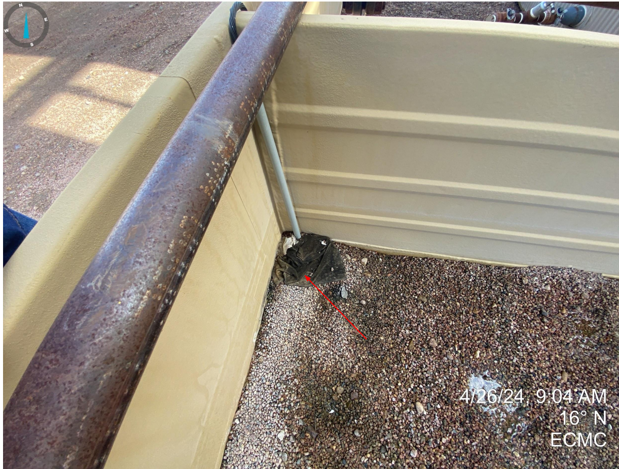
Photo 16. Oily rag observed within tank battery secondary containment.
