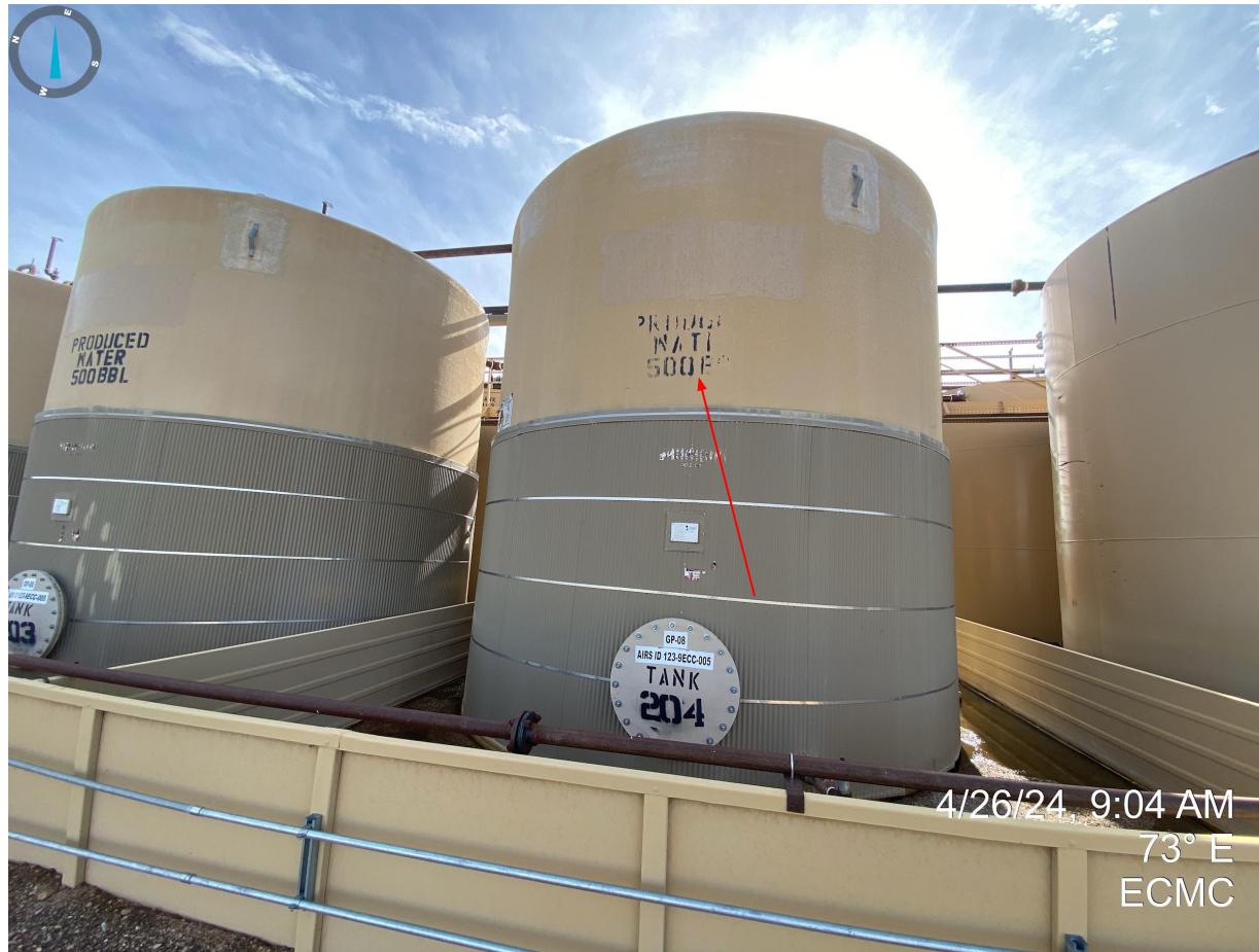
Photo 15. Tank labels/NFPA placards are faded, peeling, cracked.
