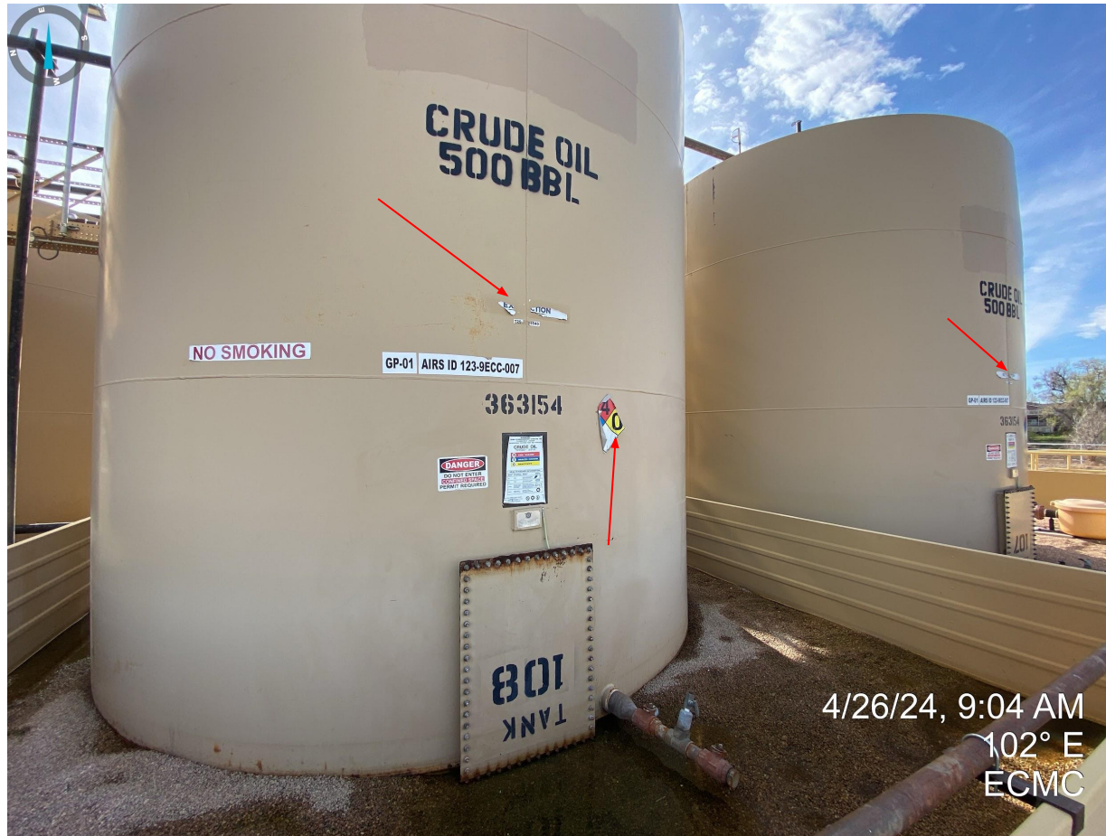
Photo 14. Tank labels/NFPA placards are faded, peeling, cracked.
