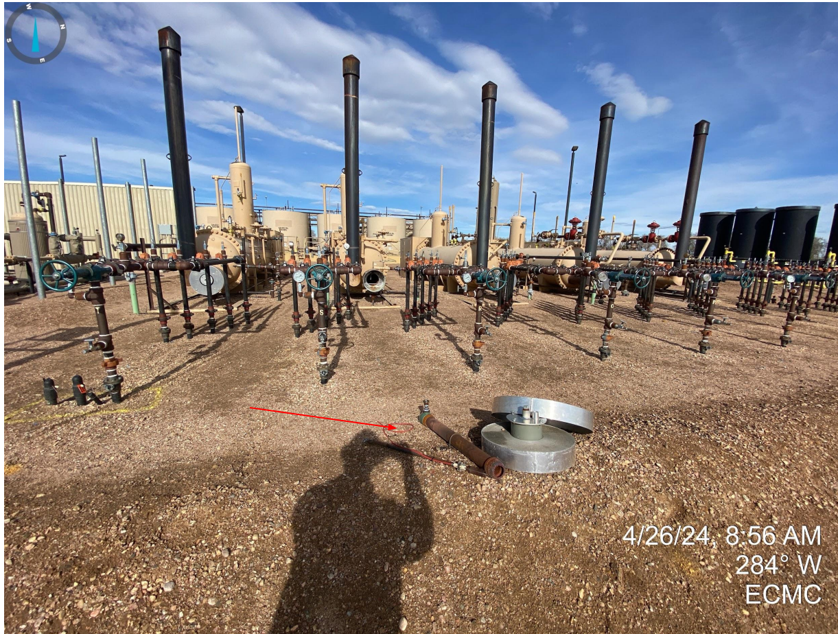
Photo 1. Unused equipment must be removed or returned to service.
