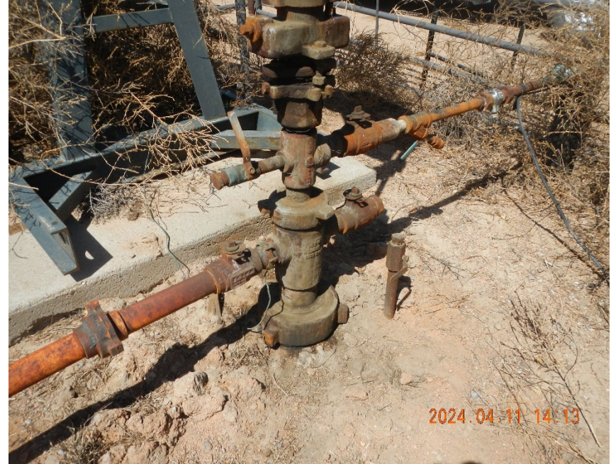
6. Additional view of wellhead.
