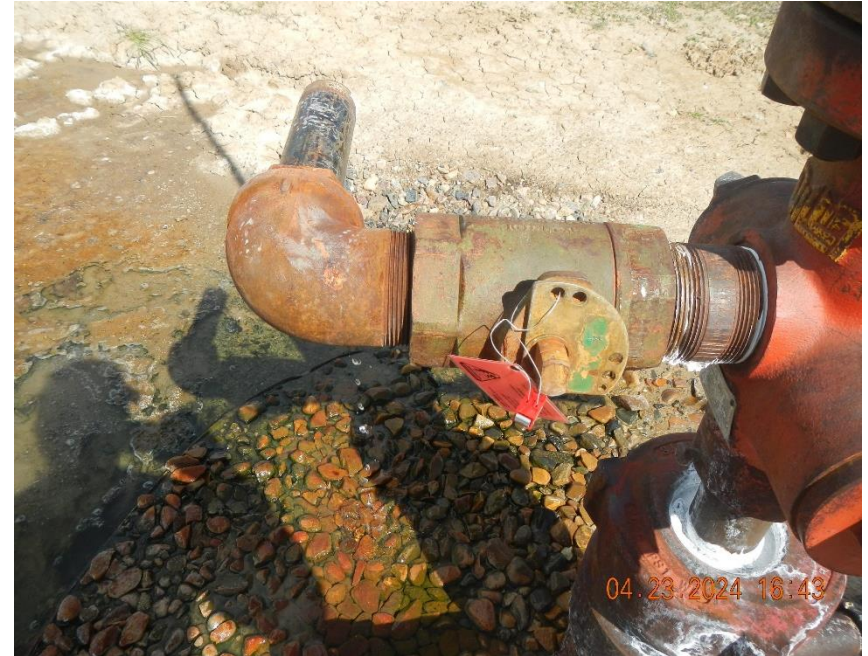
BLM tag on 2 inch valve. Valve is broken and leaking.
