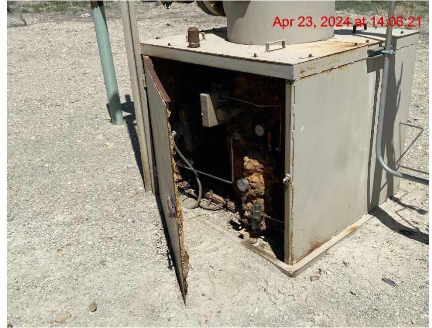
Unsecured Hatch/Wildlife Entry Hazard – Photo #00791
