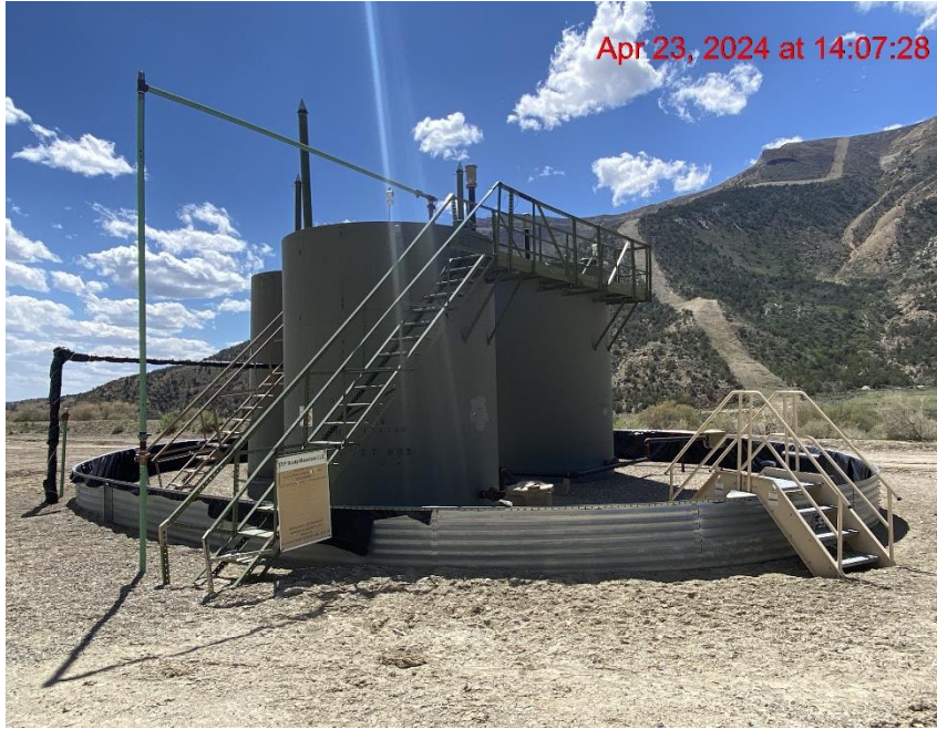
Tank Battery – Photo #00794
