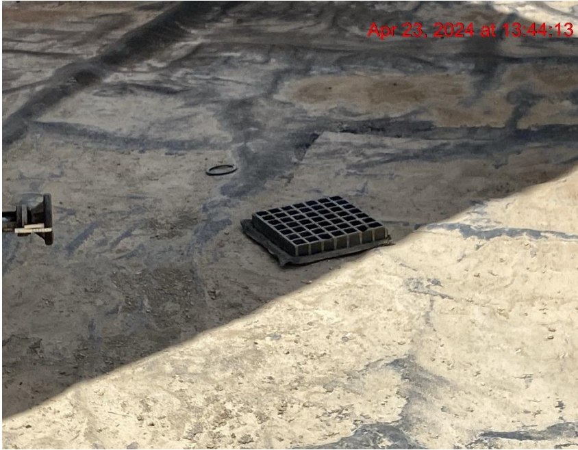
Debris in Secondary Containment – Photo #00771
