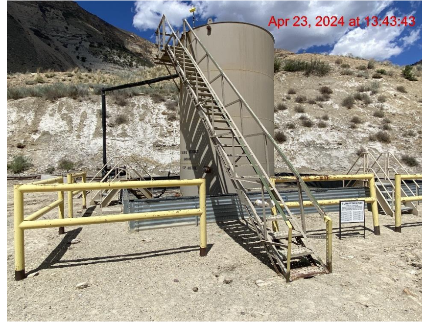
Tank Battery – Photo #00768
