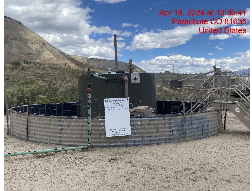
Tank Battery – Photo #00742
