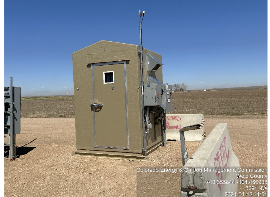
Photo #8 CVR Pad/5-63-32 Battery site Active Instrument Air Unit(s)
