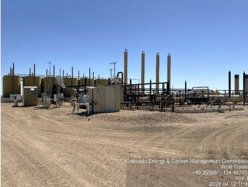
Photo #1 CVR Pad/5-63-32 Battery site Active
