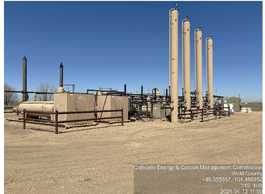
Photo #6 CVR Pad/5-63-32 Battery site Active Separator(s), VRT(s), VRU(s)
