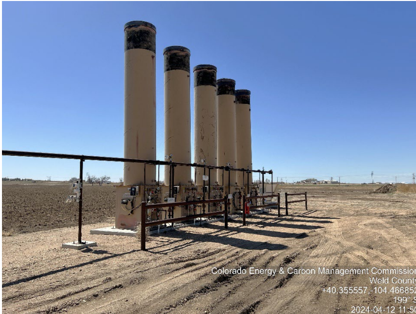
Photo #5 CVR Pad/5-63-32 Battery site Active ECD(s)
