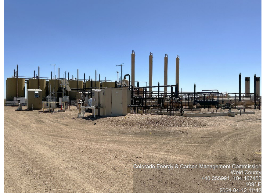
Photo #10 CVR Pad/5-63-32 Battery site Active Equipment Documented; Loc ID: 432011
