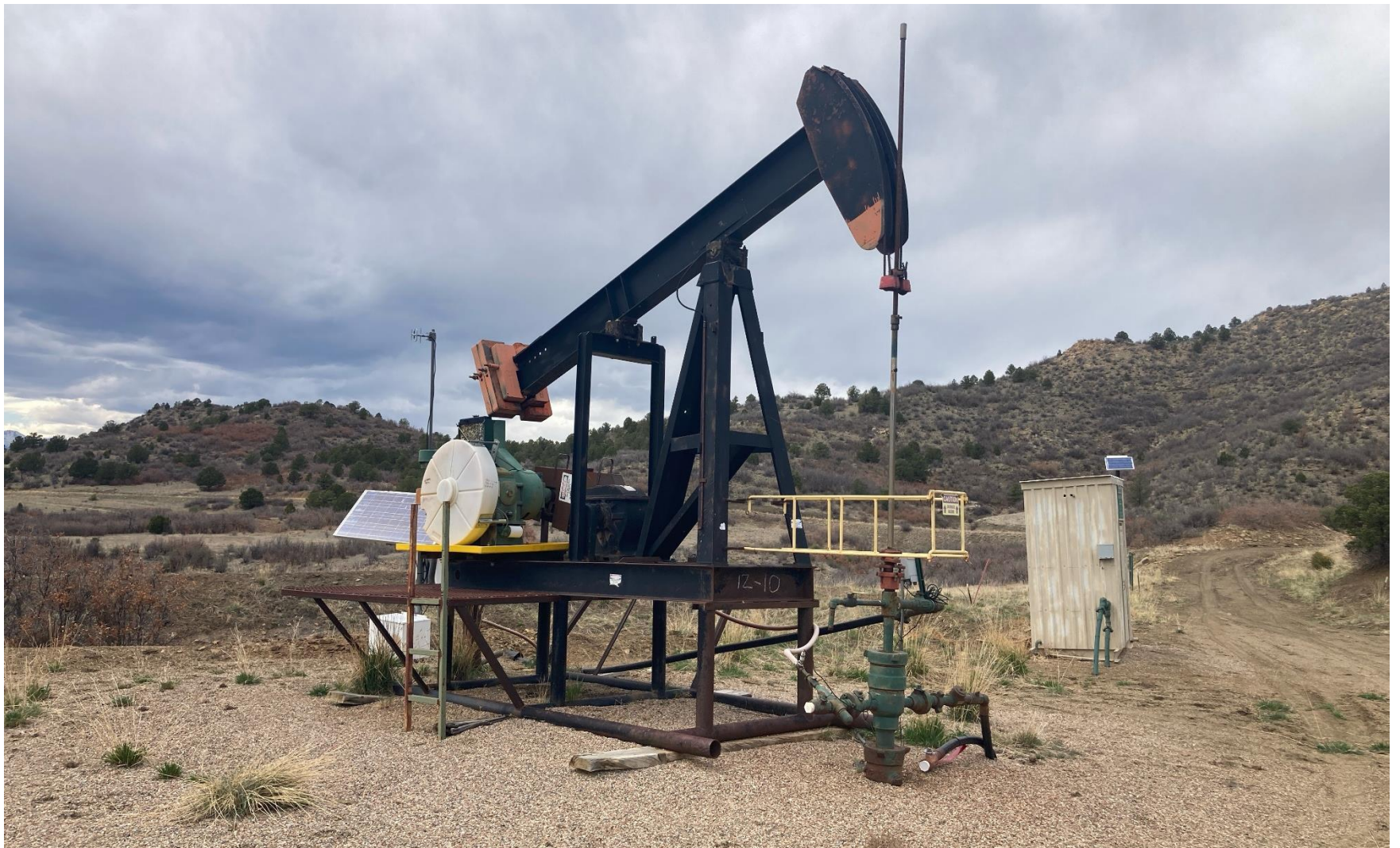
PHOTO 3: WELLHEAD AND EQUIPMENT
