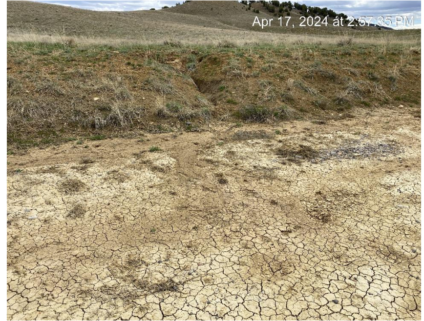
Erosion and sediment migration entering location
