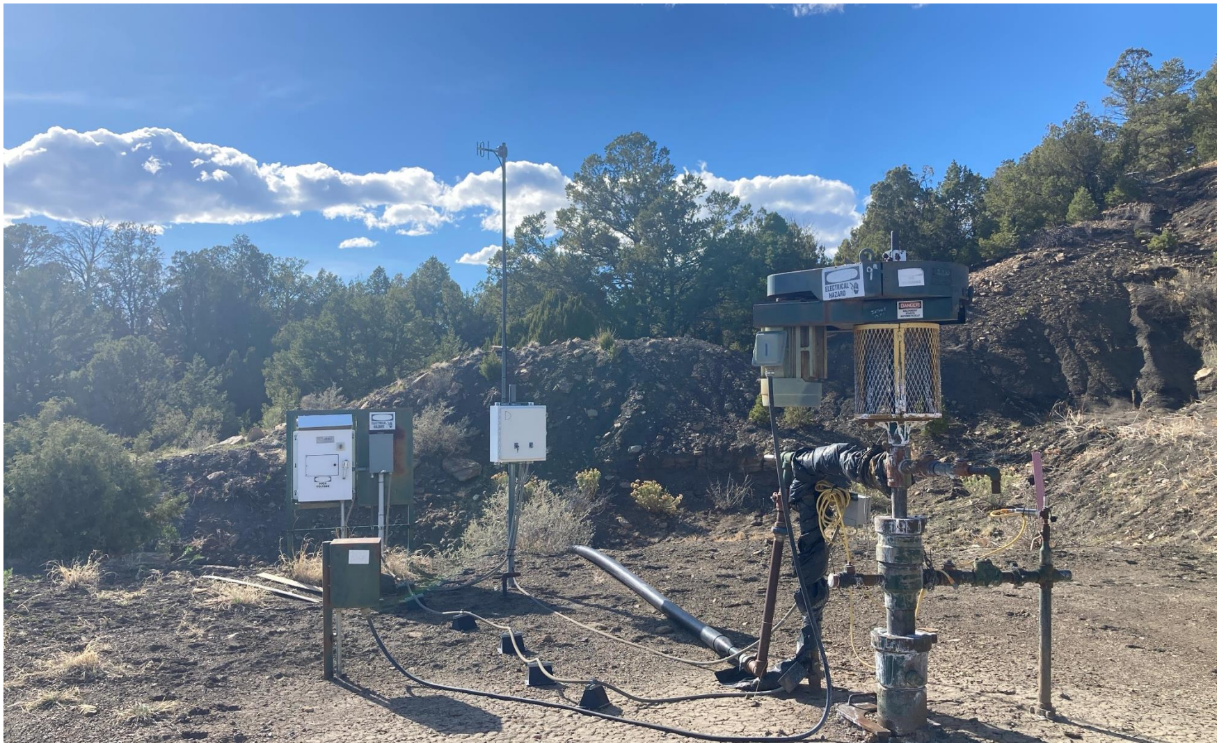
PHOTO 3: WELLHEAD AND EQUIPMENT
