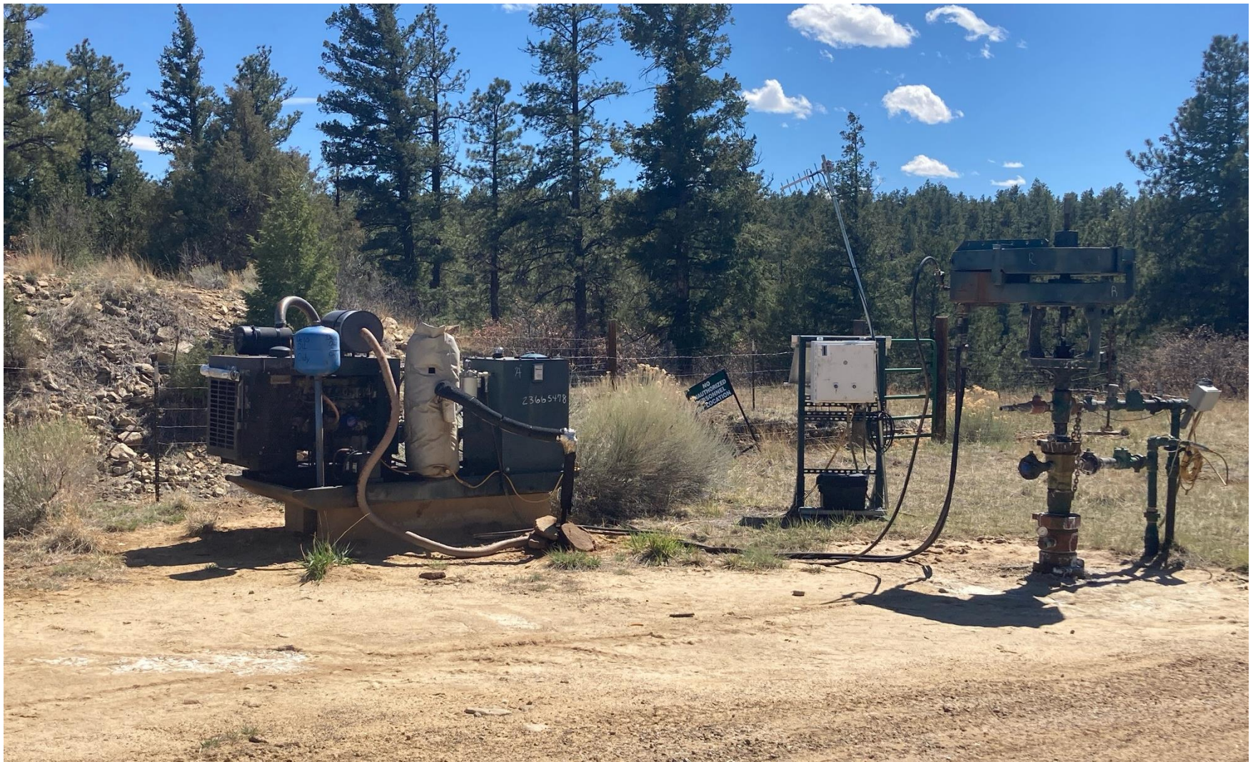
PHOTO 3: V WELLHEAD AND EQUIPMENT
