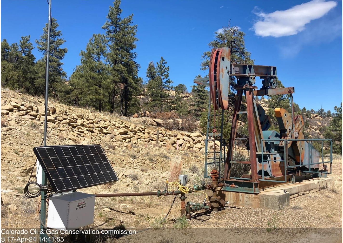
PHOTO 4: R WELLHEAD AND EQUIPMENT
