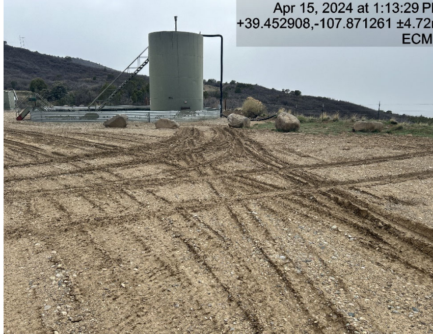
Areas of lack of stabilization/compaction
