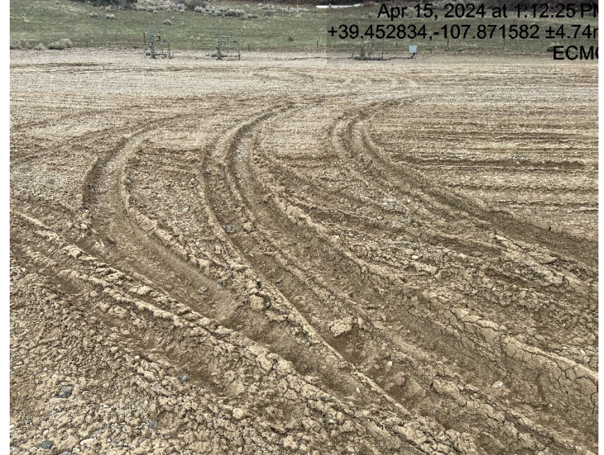
Areas of lack of stabilization/compaction
