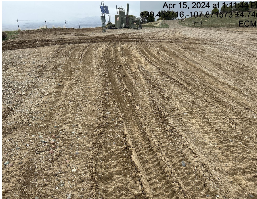
Areas of lack of stabilization/compaction
