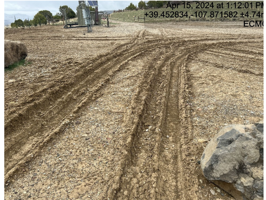
Areas of lack of stabilization/compaction
