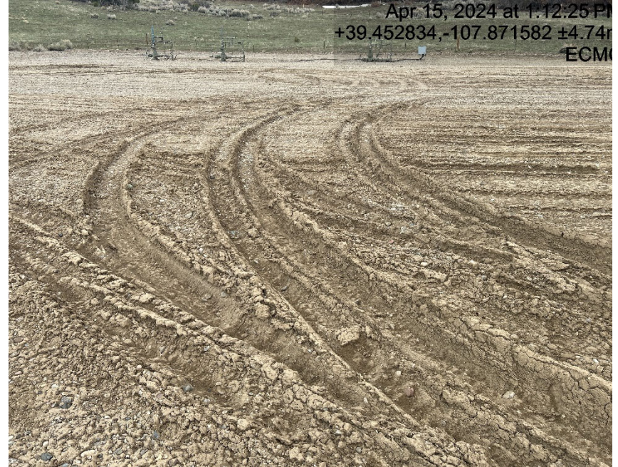
Areas of lack of stabilization/compaction
