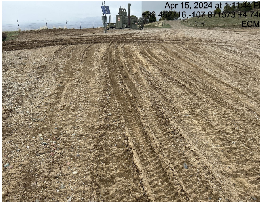
Areas of lack of stabilization/compaction
