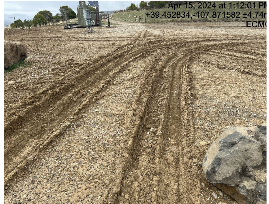
Areas of lack of stabilization/compaction
