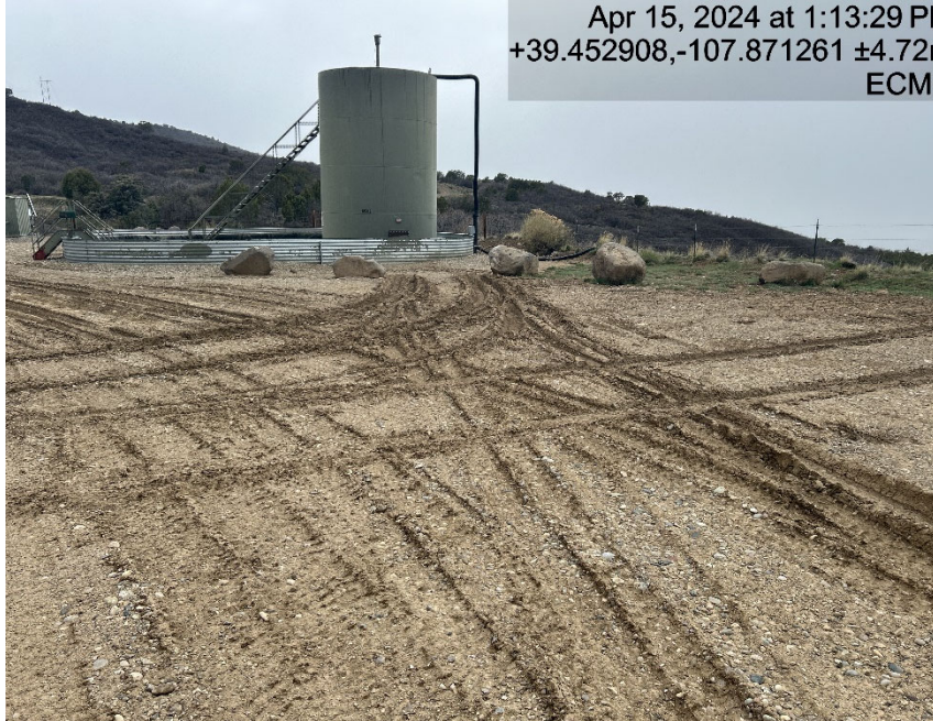
Areas of lack of stabilization/compaction
