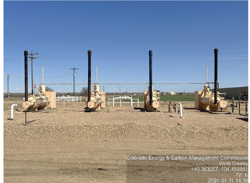
Photo #4 Siebring 41-32, 31-32, 32-32, 42-32, CNE-32 Battery site Inactive | Shut-down Separator(s)
