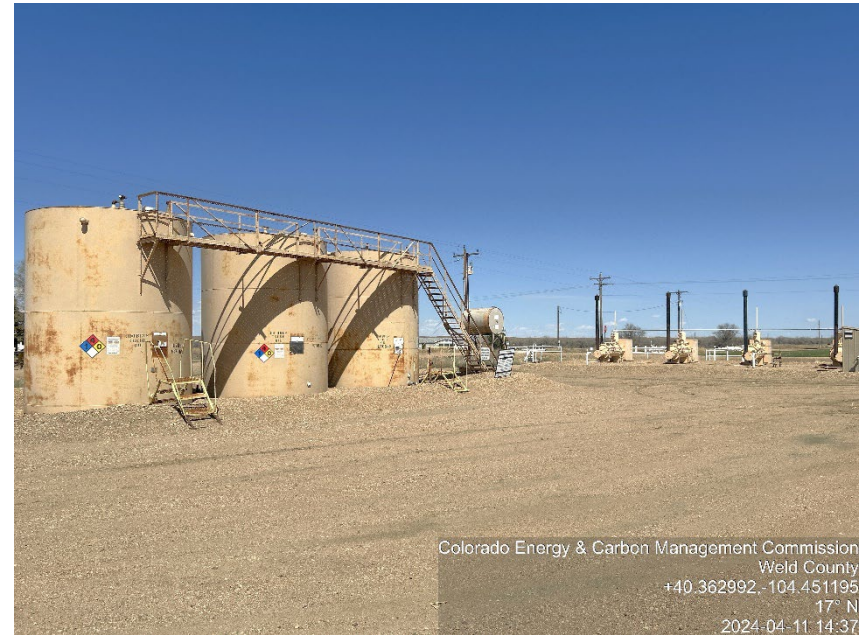
Photo #2 Siebring 41-32, 31-32, 32-32, 42-32, CNE-32 Battery site Inactive | Shut-down Equipment Documented; Loc ID: 332237
