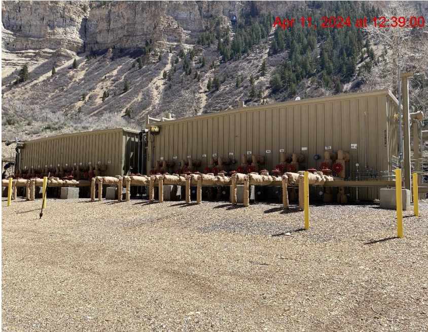
Separator Housing – Photo #00585
