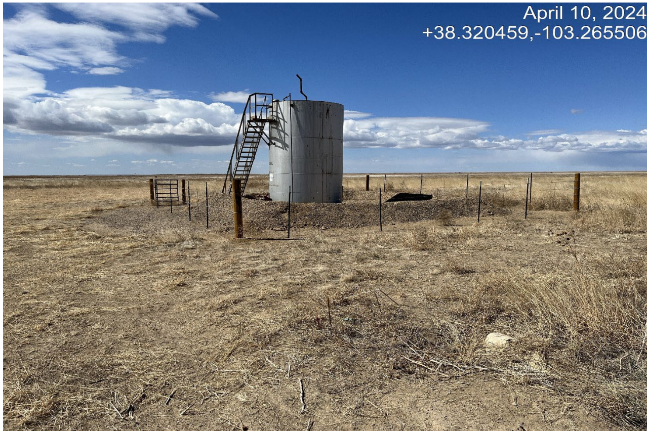
Photo 1. Facing south toward the tank battery which has been fenced and berm was rebuilt.
