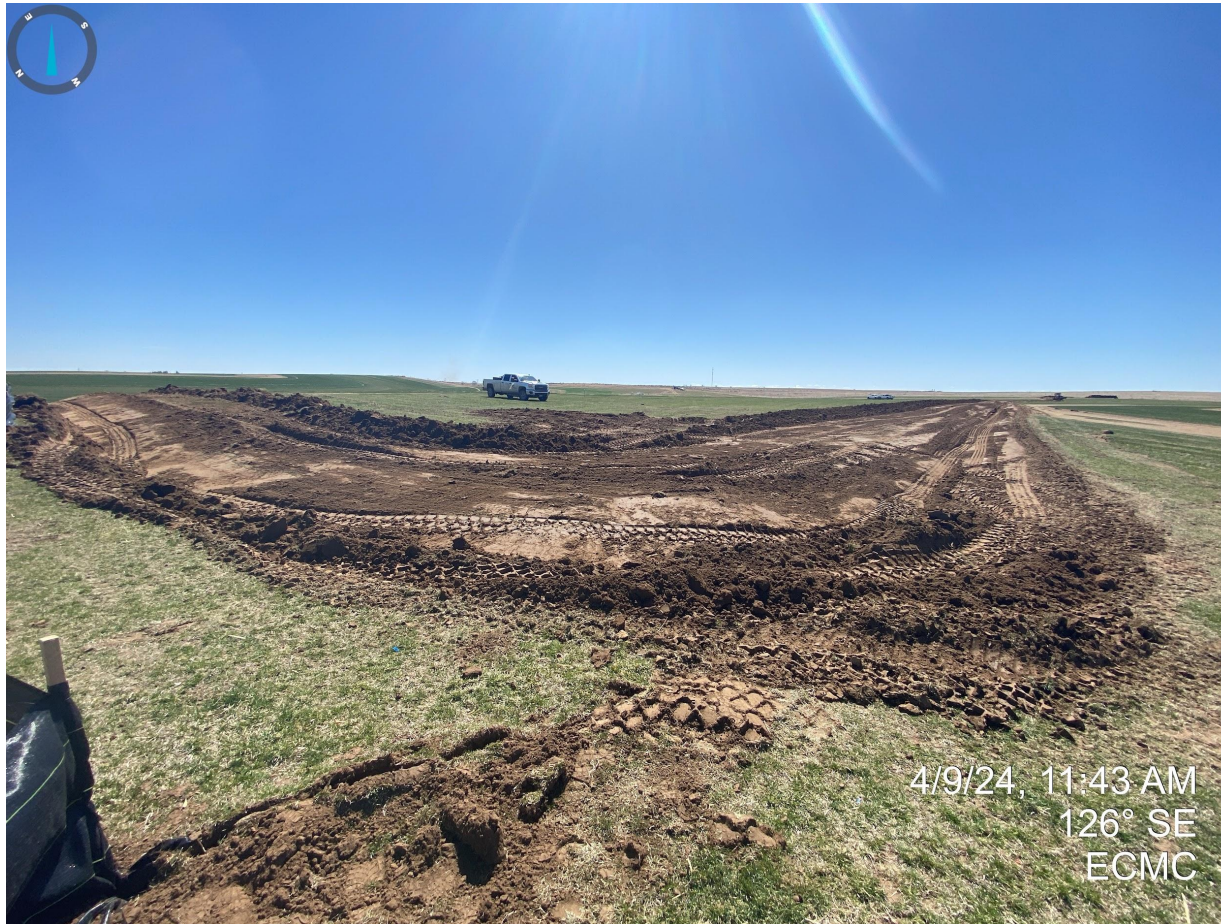
Photo 5. Taken near the northwest corner of the disturbance area. Topsoil salvage operations had not commenced at the time of this inspection; onsite crews were in the process of installing a perimeter stormwater control BMP (ditch and berm).
