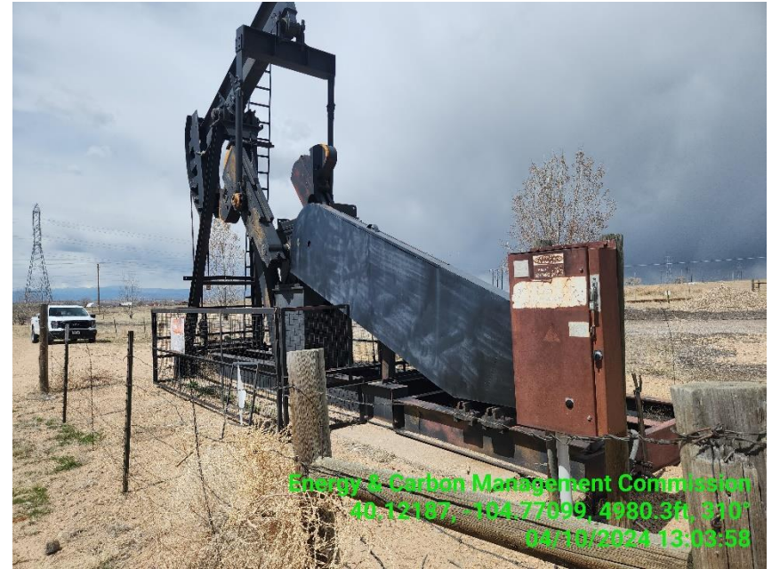
Photo 4 Pump jack & electric panel.
