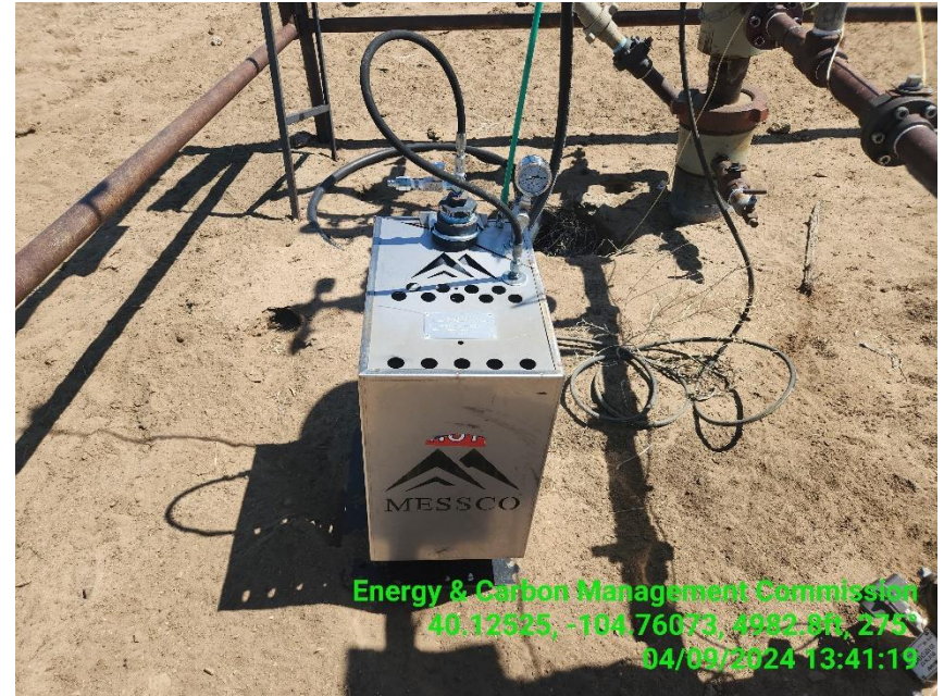
Photo 2 Fugitive gas recovery unit.
