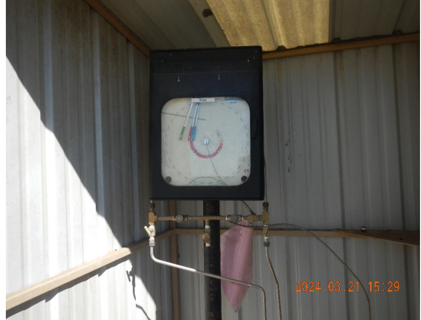
6. Gas meter inside remote meter shed.
