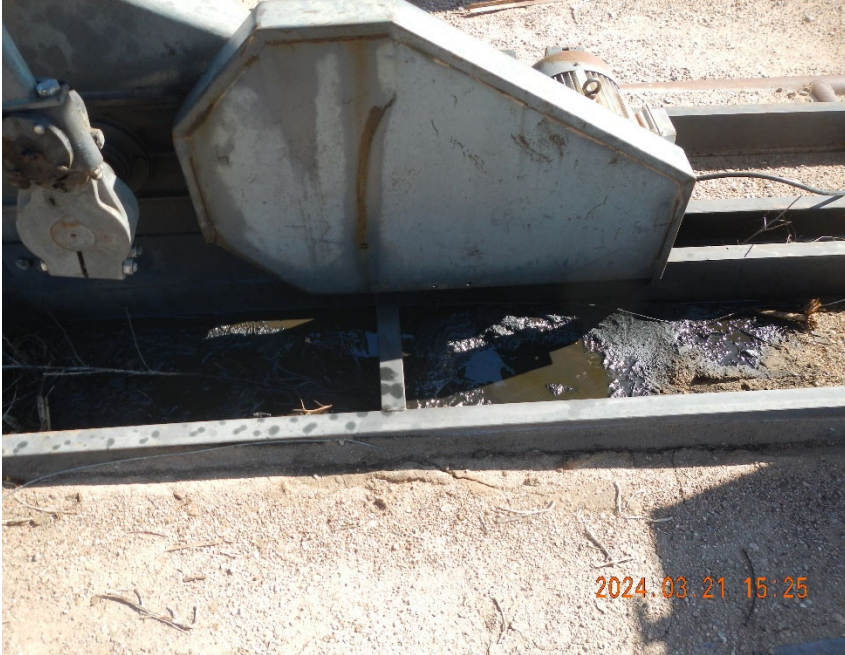
3. Stained soil under pumping unit gear reducer and prime mover.
