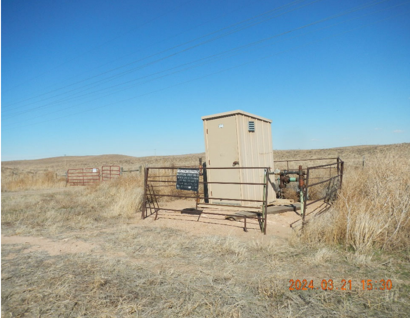
5. Remote metering location overview.
