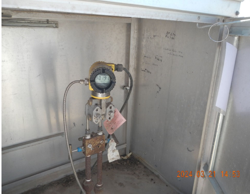
3. Digital gas meter inside meter box.
