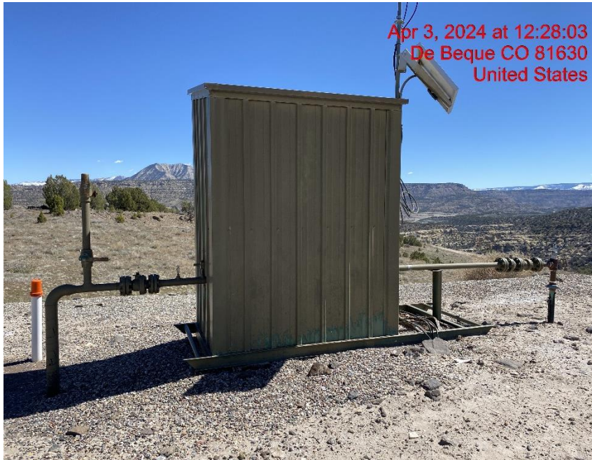
Gas Meter– Photo #00312
