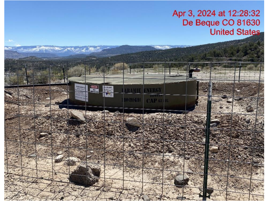
Tank Battery – Photo #00314
