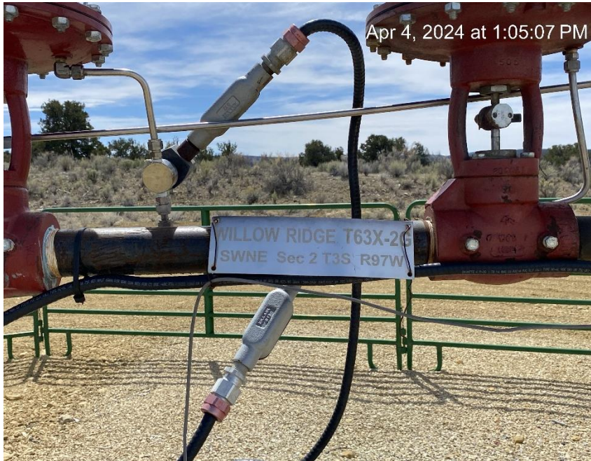
Well sign missing required information
