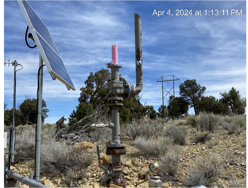
Relief riser missing rain protection
