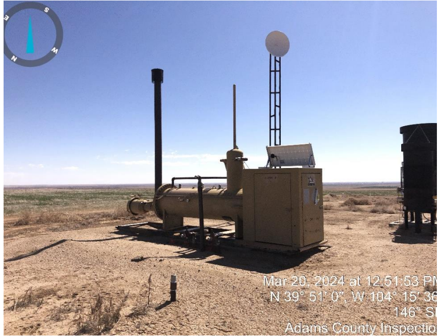
Photo #2 Separator & RTU.
