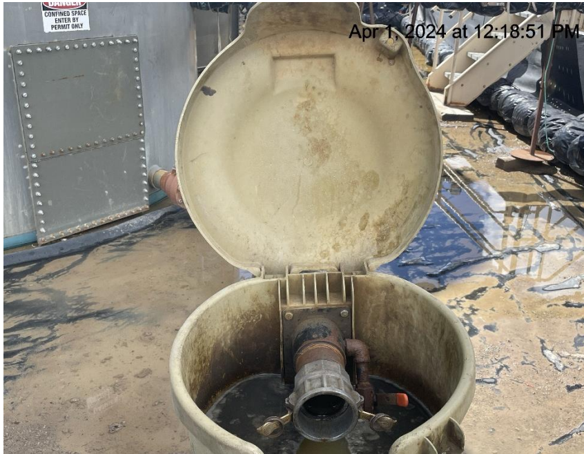
Photo # 2053 Open ended load line
