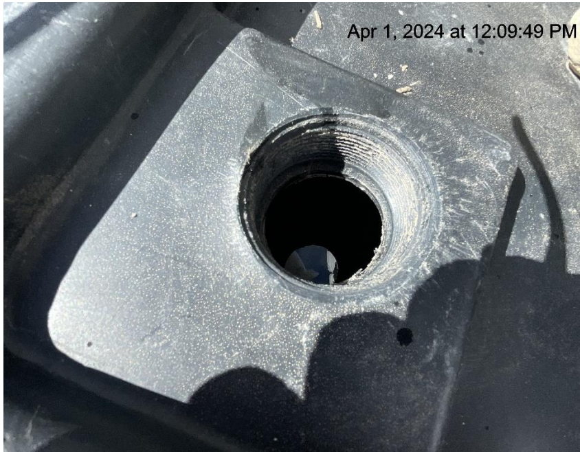
Photo # 2058 Failure to maintain chemical BMP/chemical containment approximately 3/4 full of fluid/BMP insufficient to contain possible spill.
