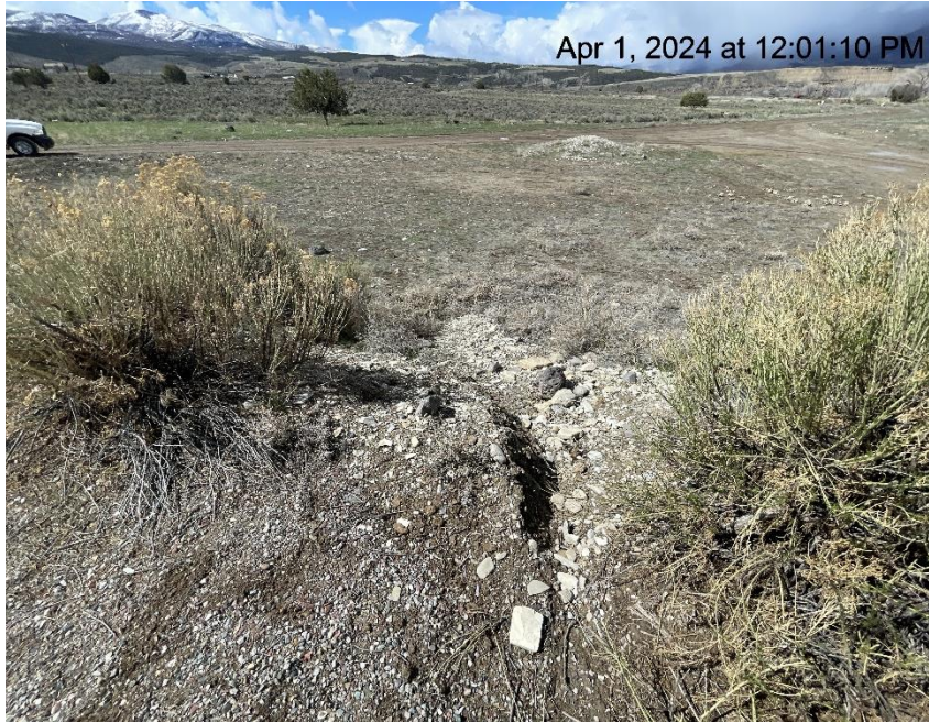
Photo # 2054 Berm/BMP needs maintenance, berm breached/eroded & sediment is being transported off location into a vegetated area. (near NW corner of location)
