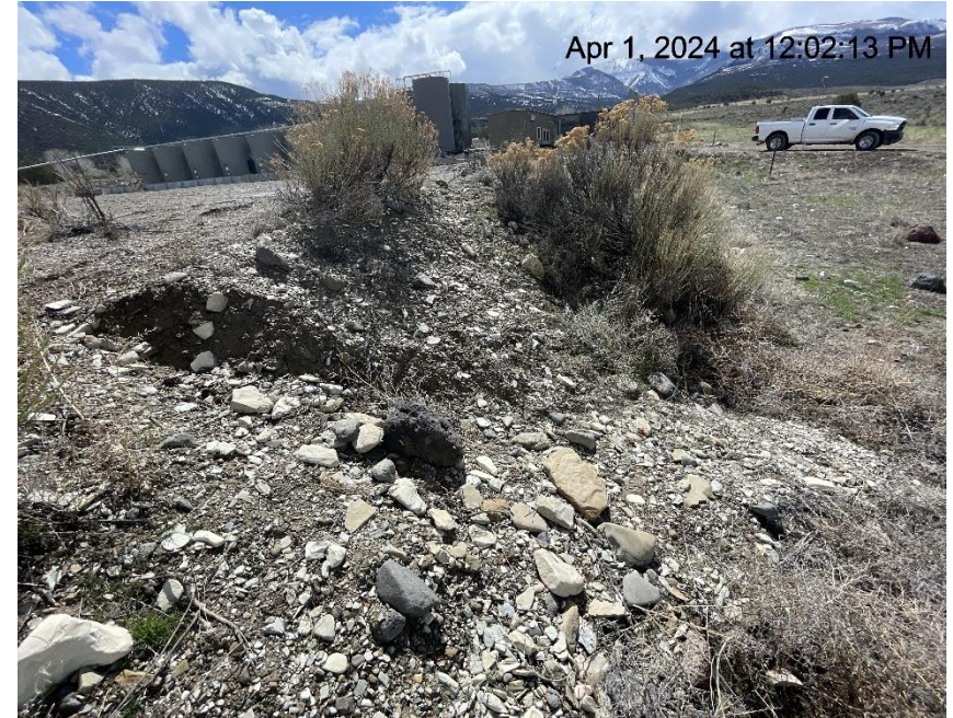
Photo # 2055 Berm/BMP needs maintenance, berm breached/eroded & sediment is being transported off location into a vegetated area. (near NW corner of location)
