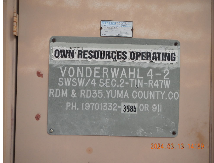
4. Well sign on remote meter shed door.
