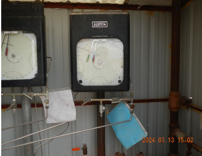
5. Gas meter inside shared meter shed.
