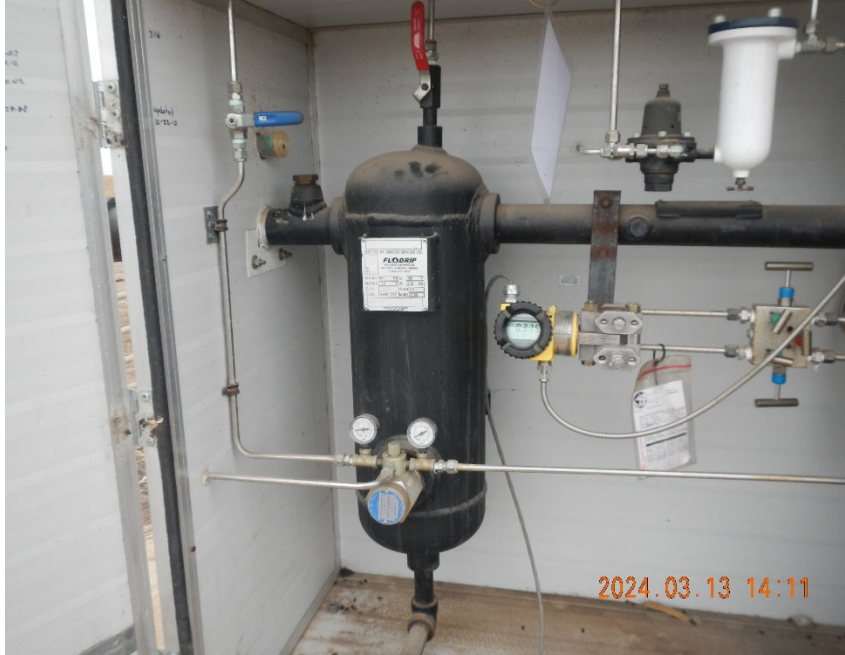
5. Separator and digital meter inside meter box.
