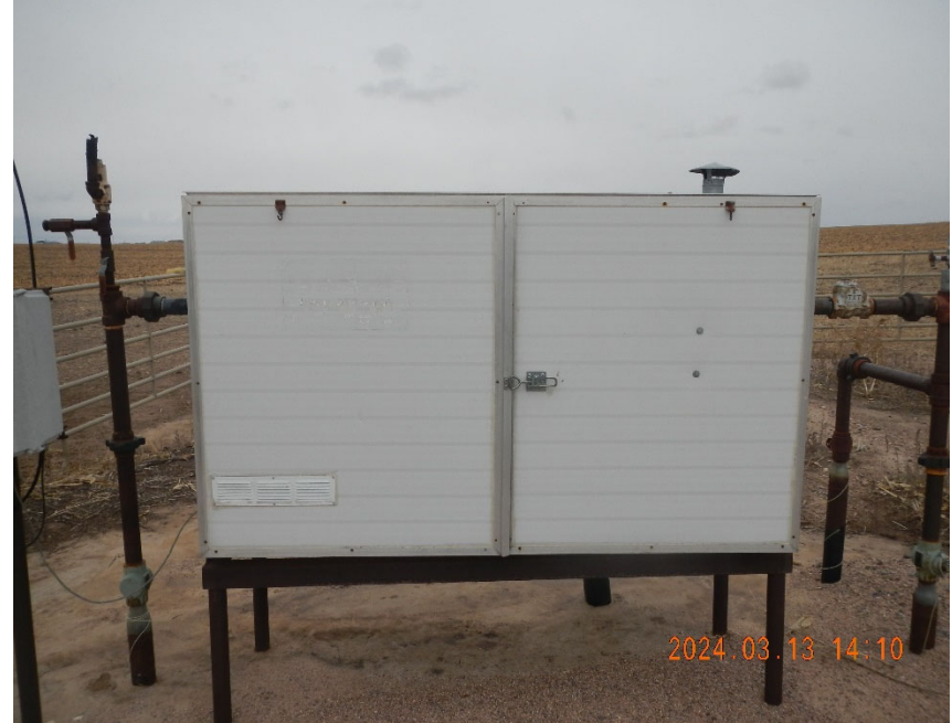
4. Remote meter box.
