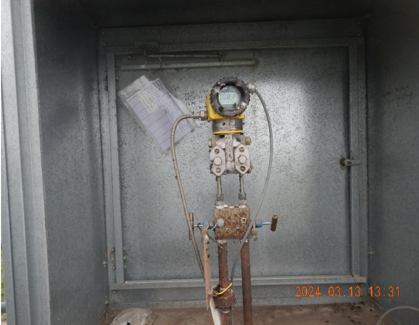
3. Digital meter inside meter box.
