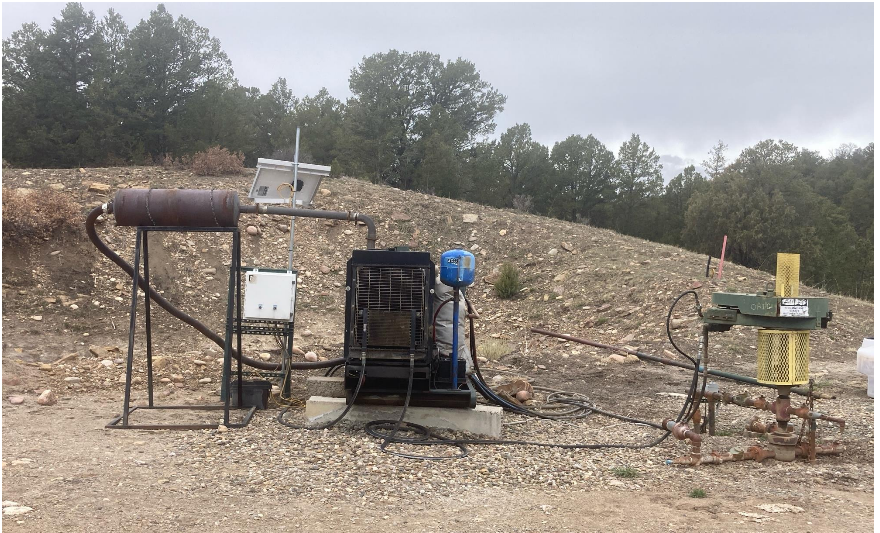
PHOTO 3: ORIG WELLHEAD AND EQUIPMENT
