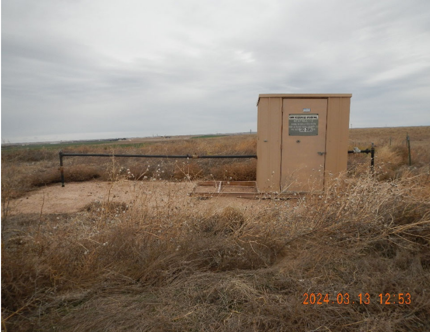
5. Remote metering location overview.
