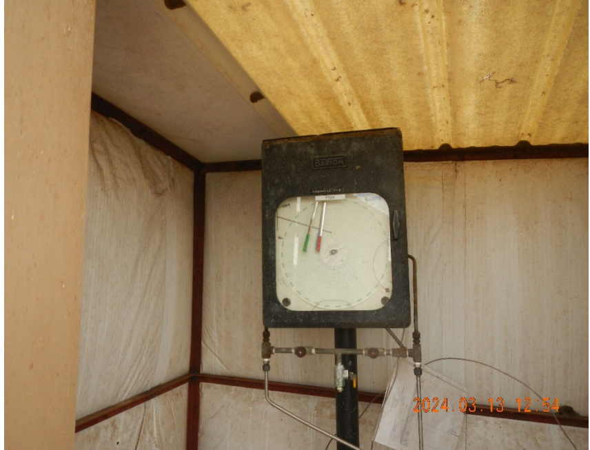
6. Gas meter inside meter shed.
