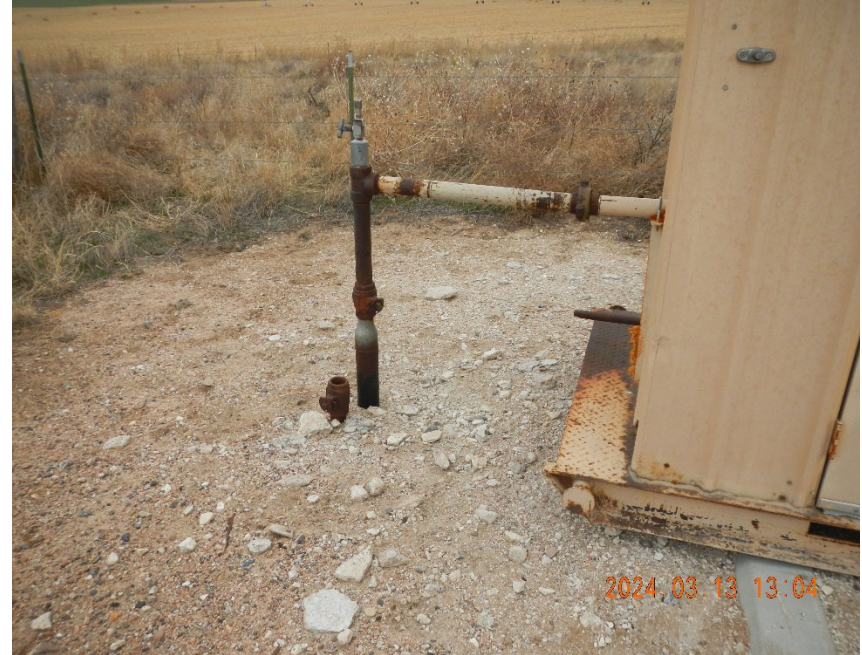
6. Flowline riser with valve at remote meter shed.
