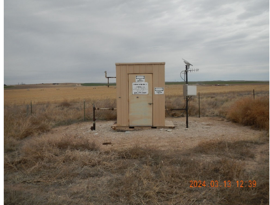
4. Remote metering location outside pivot.
