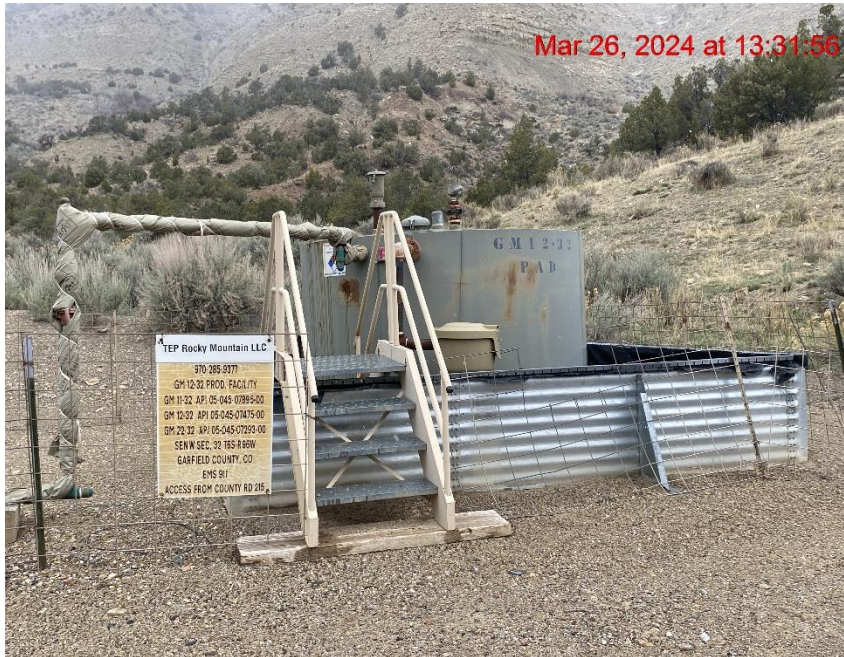
Tank Battery – Photo #00171
