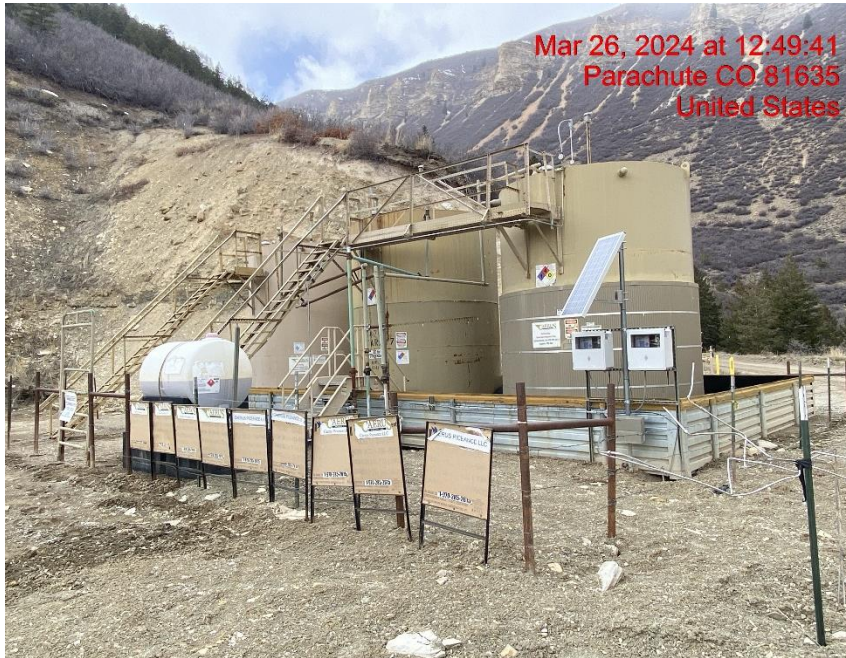
Tank Battery – Photo #00133
