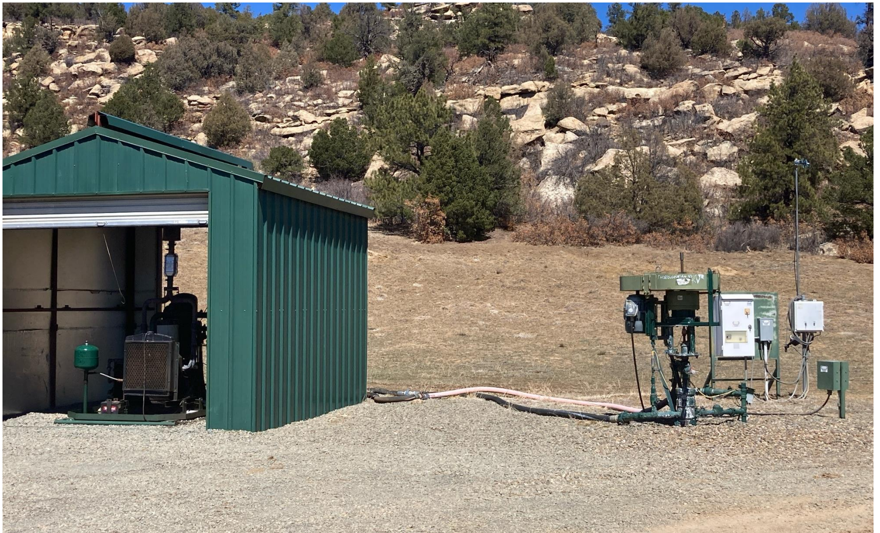
PHOTO 3: KB WELLHEAD AND EQUIPMENT
