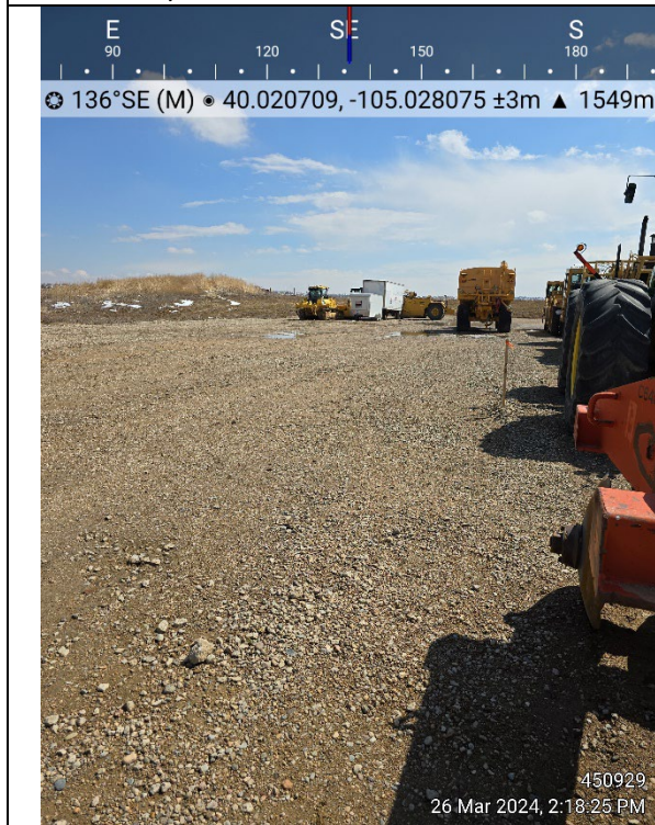
Looking Southeast at equipment on MLVT Pad – 40.020709 / -105.028075
