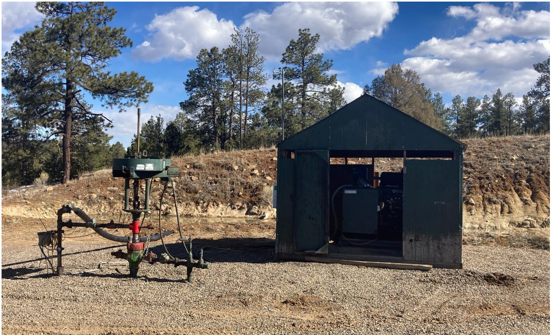
PHOTO 3: ORIG. WELLHEAD AND EQUIPMENT
