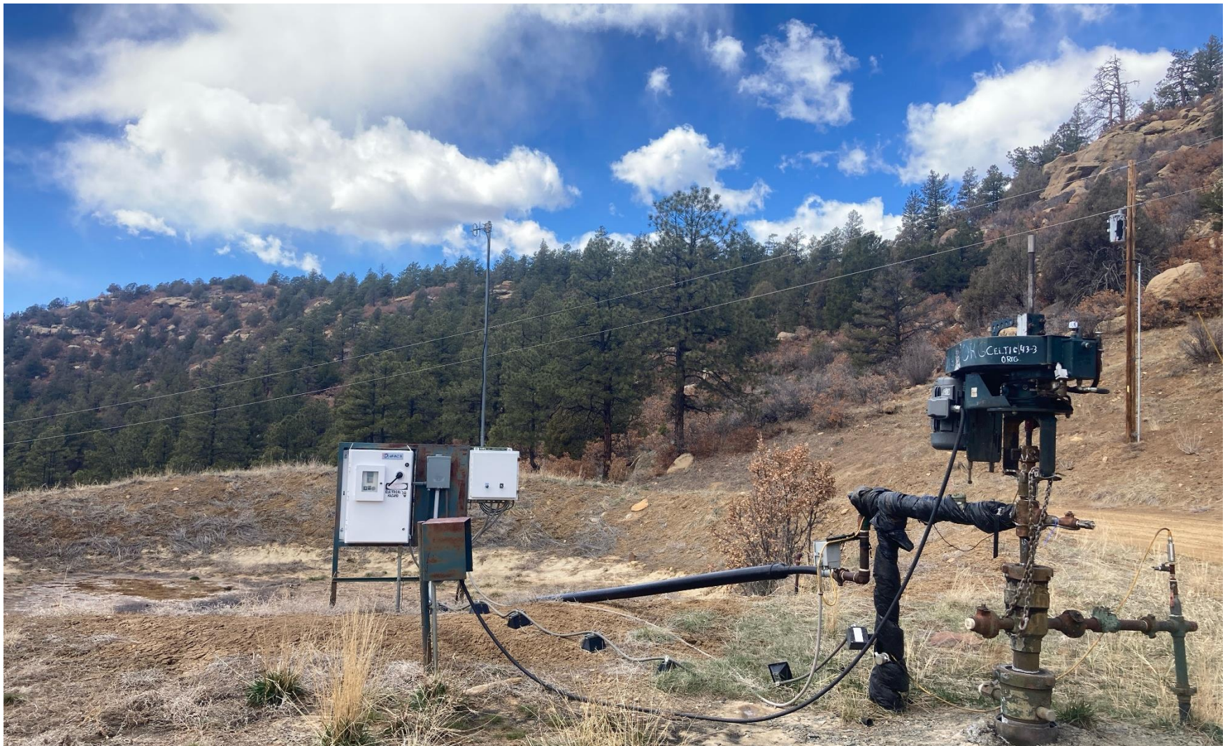
PHOTO 3: ORIG. WELLHEAD AND EQUIPMENT
