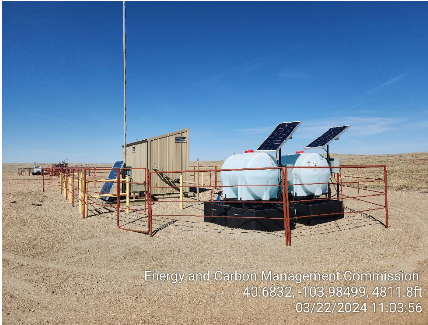
Photo 5 – Gas Lift Injection Meter House
