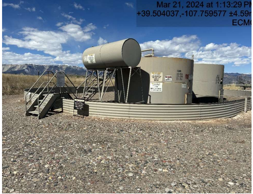
Location and battery signage lacking information
