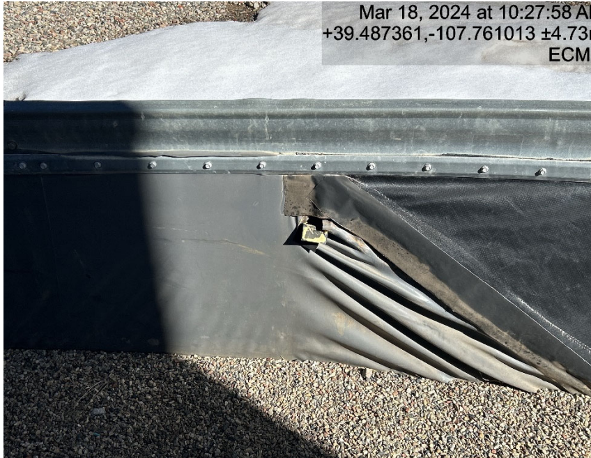
Hole in secondary containment
