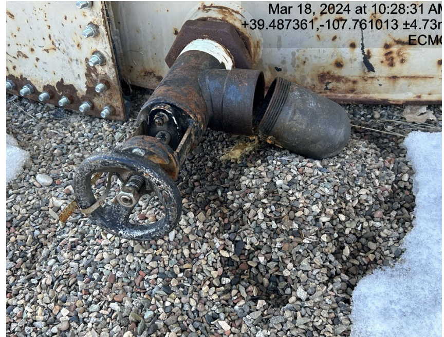
Leaking valve and cap not installed properly
