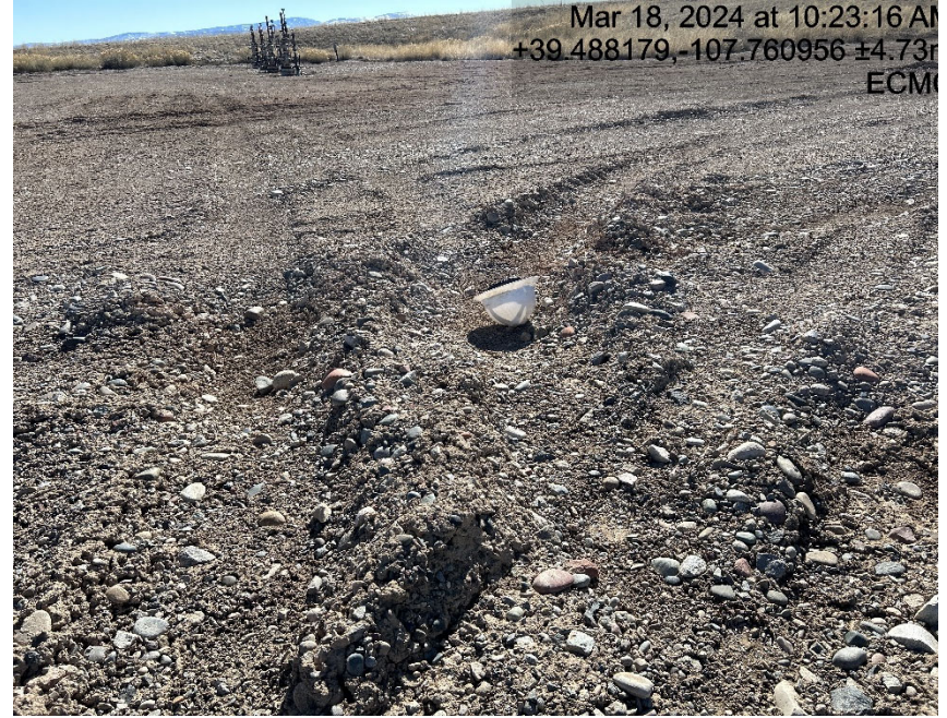
Lack of stabilization/ compaction
