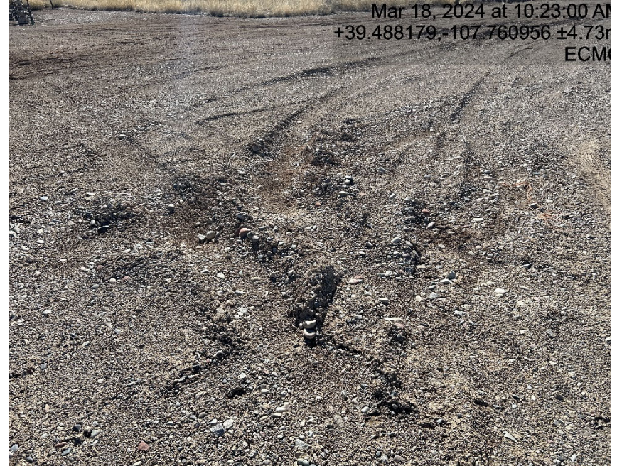
Lack of stabilization/ compaction
