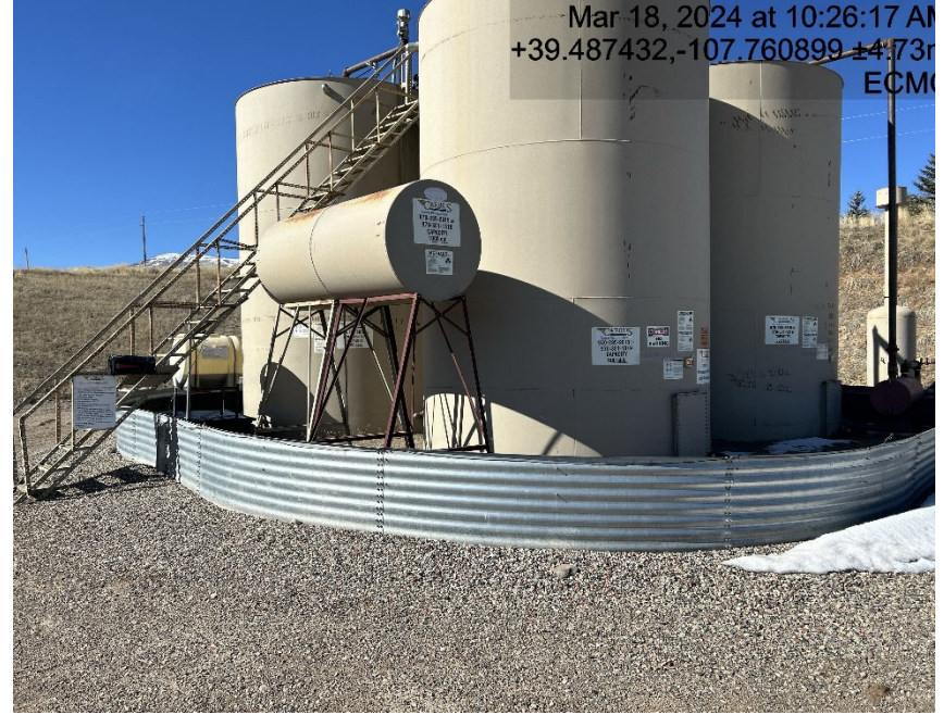
Lack of tank battery signage
