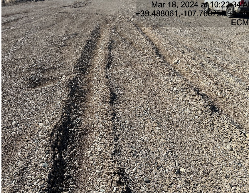
Lack of stabilization/ compaction
