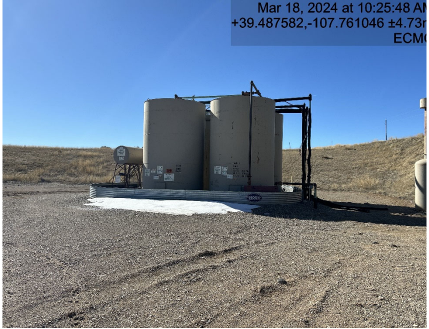
Lack of tank battery signage
