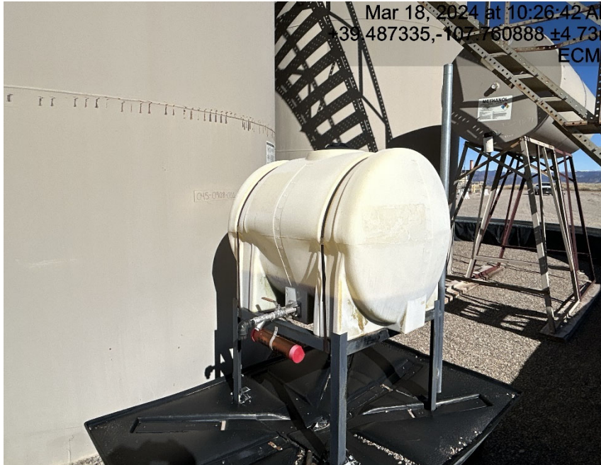
Labeling is illegible
