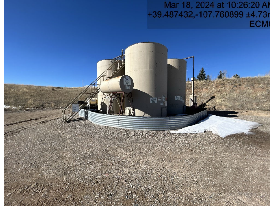
Lack of tank battery signage
