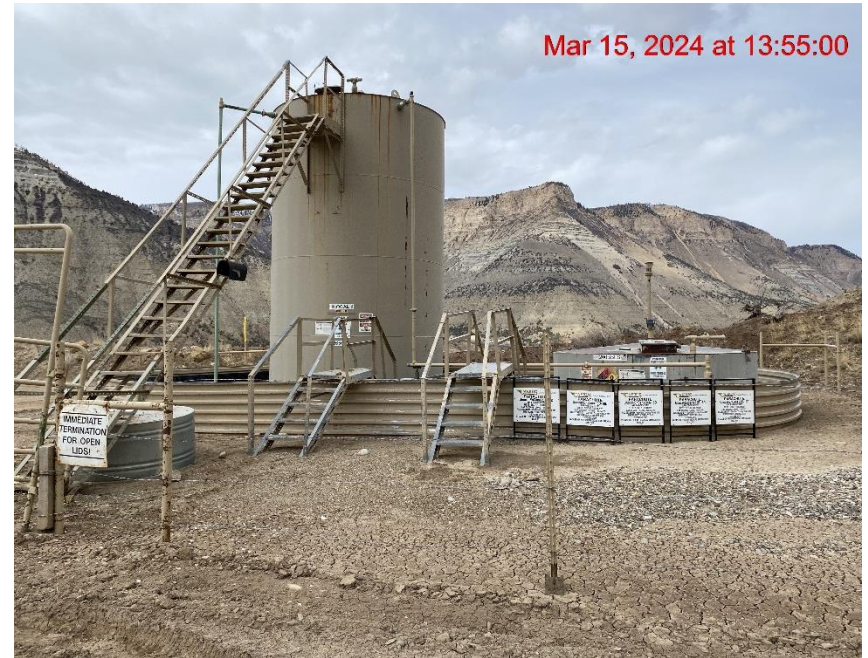
Tank Battery – Photo #09991
