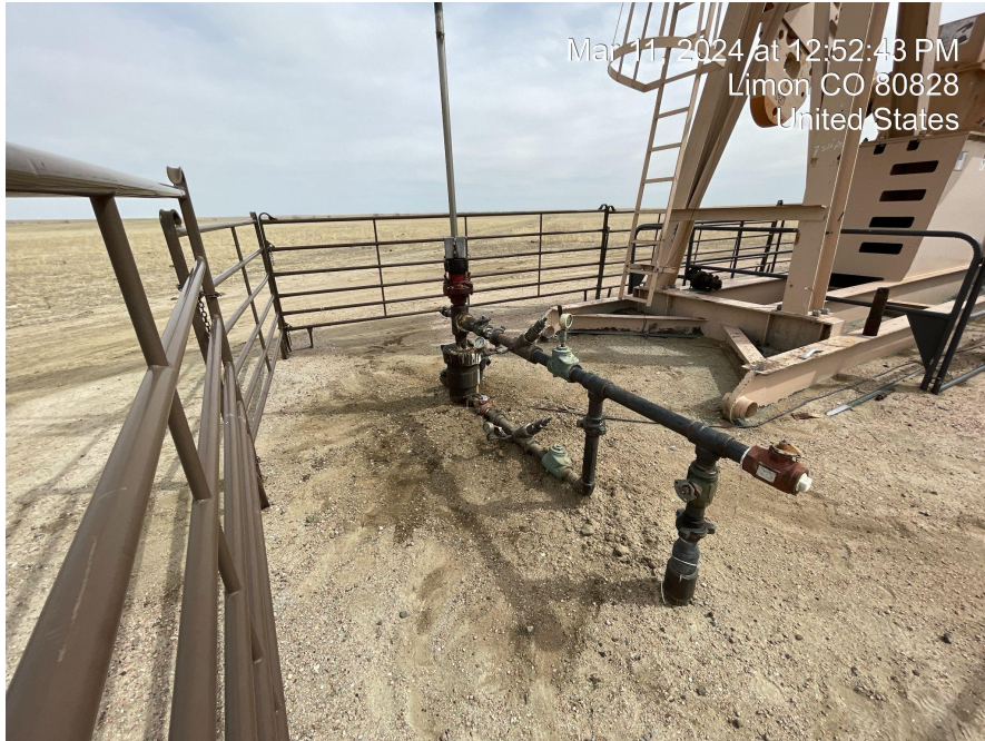
Photo 3. Photo taken facing northeast of staining around wellhead.
