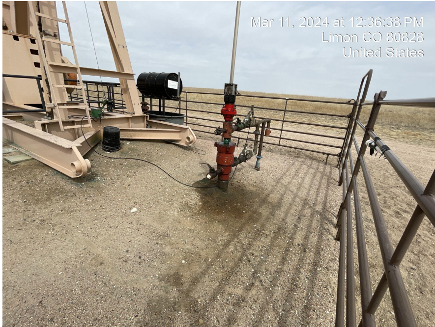
Photo 3. Photo taken facing east of staining around wellhead.
