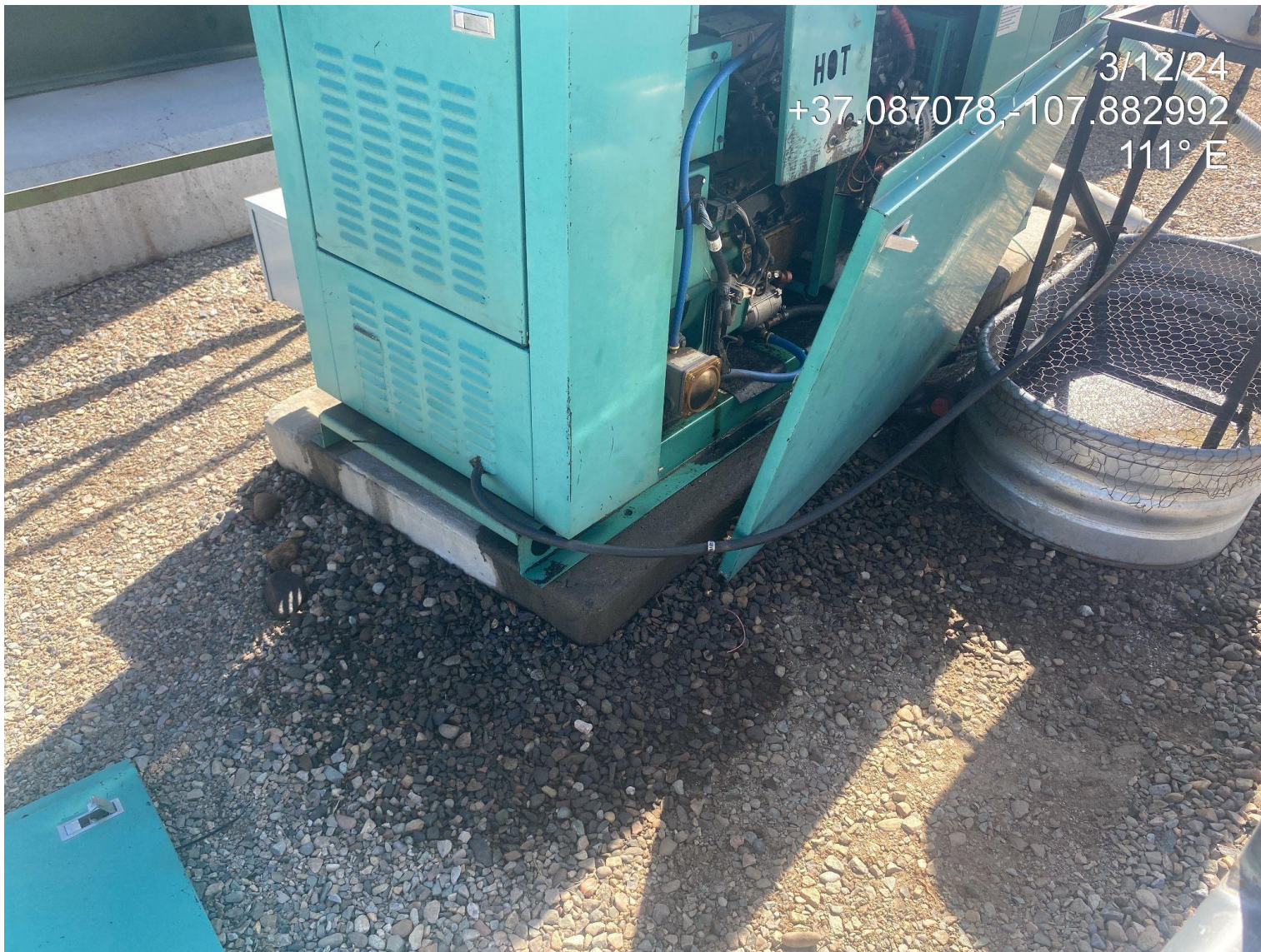
Photo 4. View of impacted surface material at the compressor.
