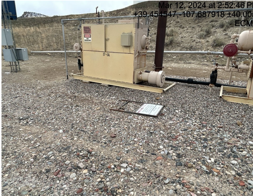
Signage on ground
