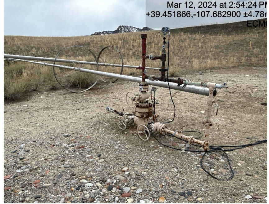
Farm equipment up against well head
