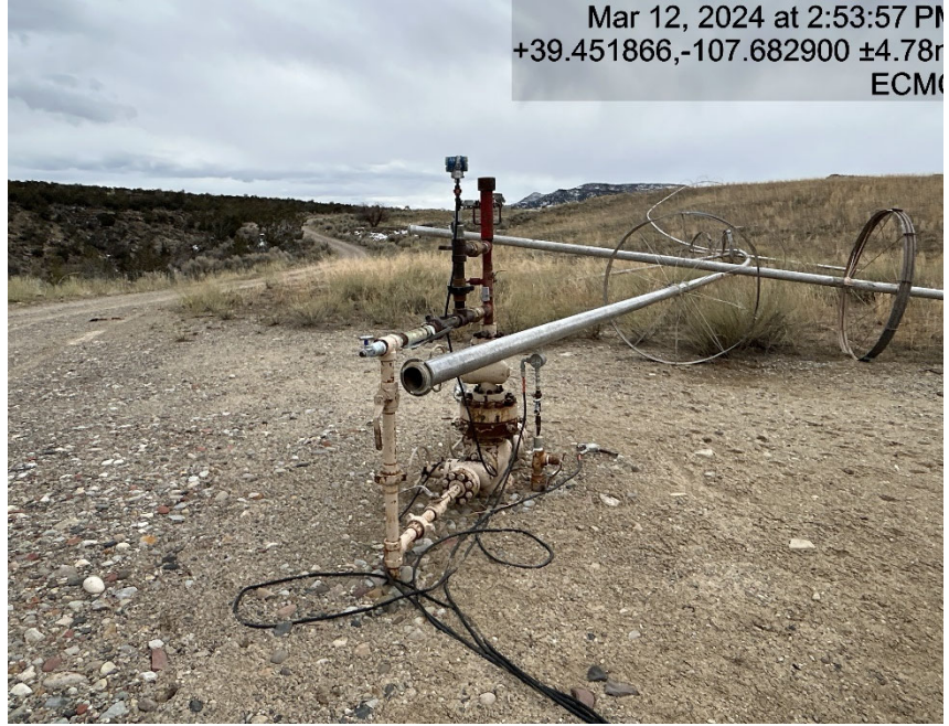
Farm equipment up against well head
