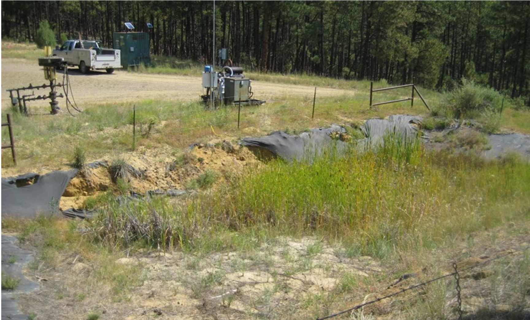
2. Silverland 31-22 Torn Pit Liner
