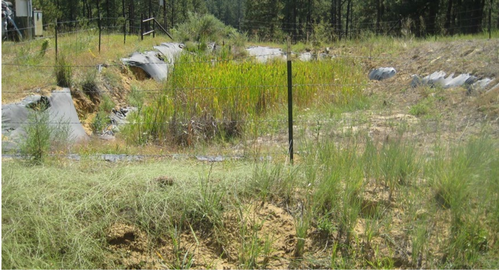
1. Silverland 31-22 Torn Pit Liner
