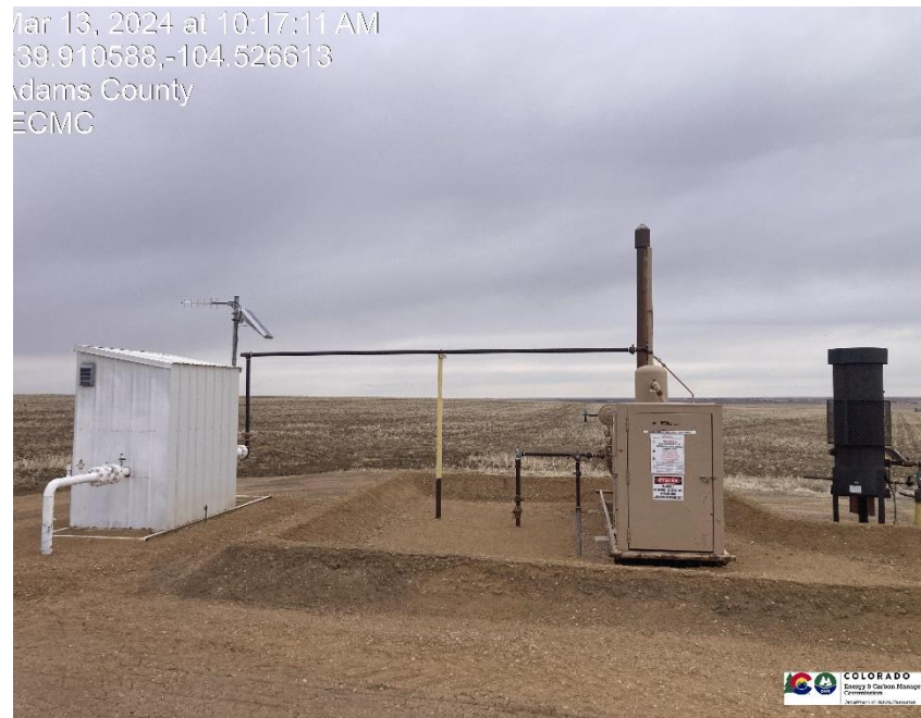
Pic 2 ECD, Separator, GMR
